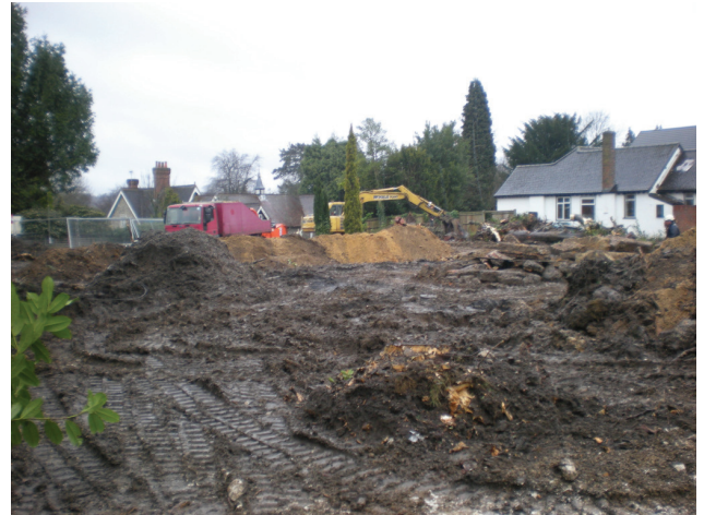
DP 4. Plot No. 8 after demolishing the house and during the evaluation. View SW.
