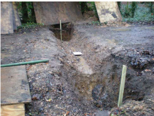
DP 5. Trench for a new drainage at NE gate of the farm. View SE.
