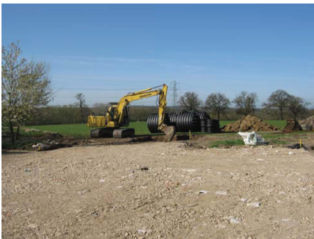
DP 9. Location of Trench 2 for sewage tank. S part of the site. View SW.
