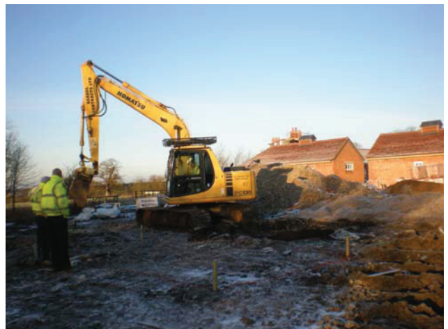
DP 6. Location of Trench 1 for sewage tank. S part of the site. February 2010. View N.
