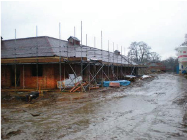
DP 1. Lower Woodside Farm, Hatfield. E part of the site. December 2009. View N.
