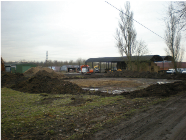
DP 1. Lower Woodside Farm, Hatfield. Area of the proposed new N barn. View S.
