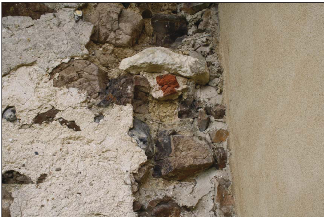
8 Putlog hole (P2) in Bay 3 north nave wall, taken from the north (41)
