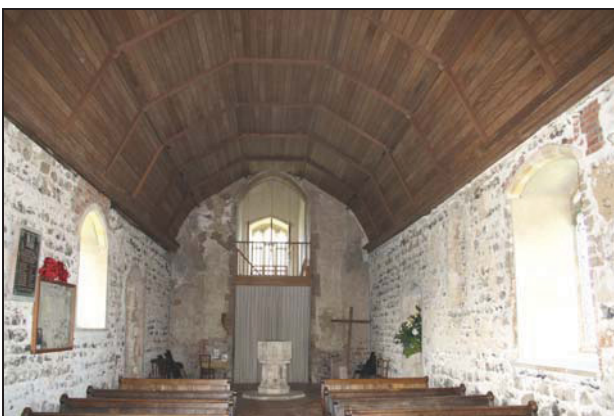
47 General view of the nave looking towards the tower, taken from the east
