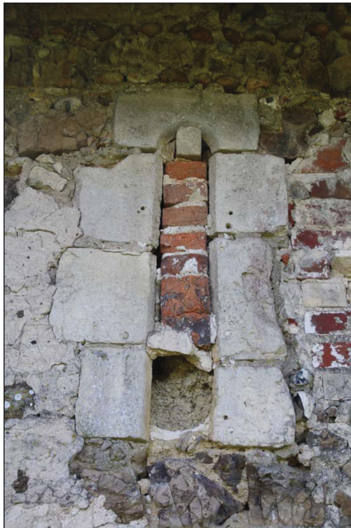
7 Detail of original lancet window in Bay 3, north nave wall, taken from the north (43)
