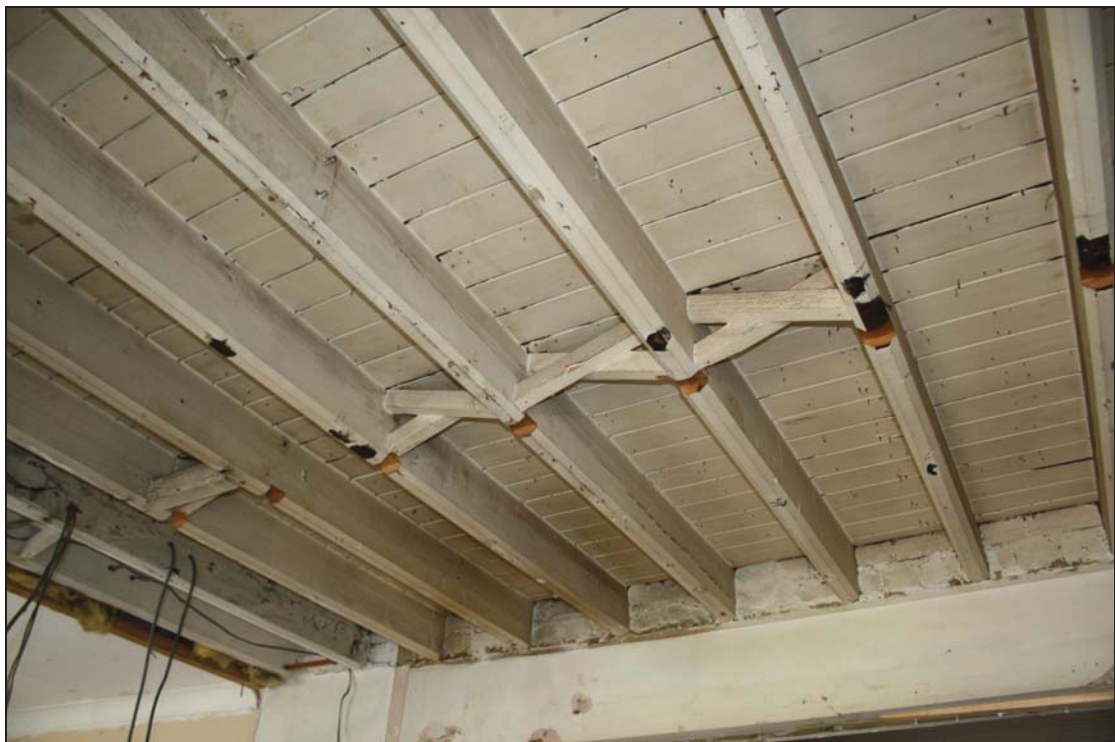
6 Detail of ceiling form showing laced bracing in Area 1 (Range 1, lower level), taken from the north (26)
