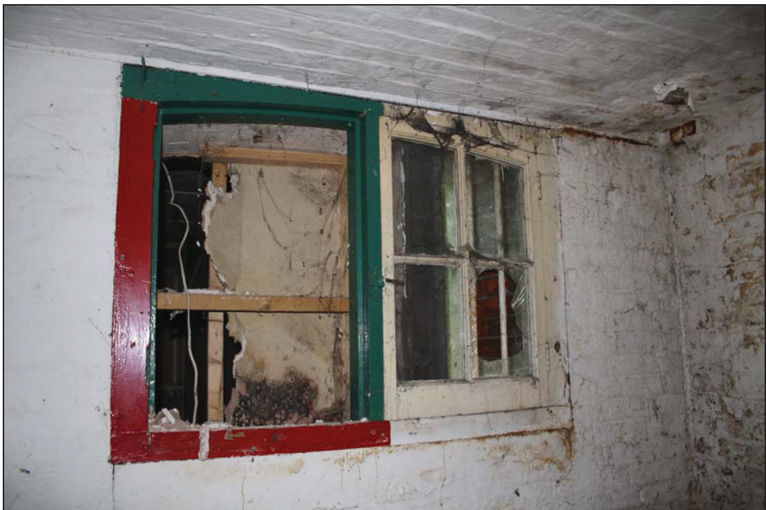
8 Original window in the formerly external south wall of Range 3, lower level, taken from the north-east (10)
