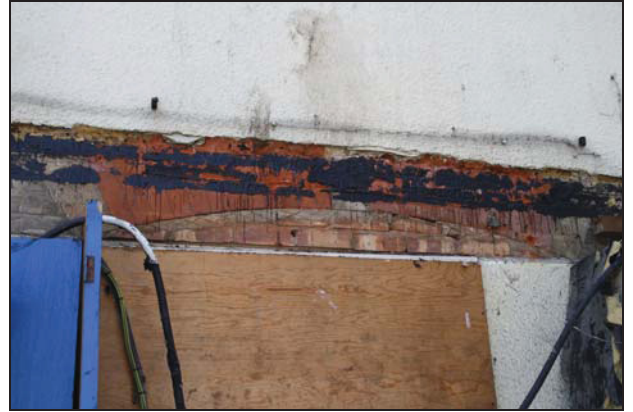
44 Arch for an original aperture on the north facade of Range 1, aperture now reduced in size, taken from the north
