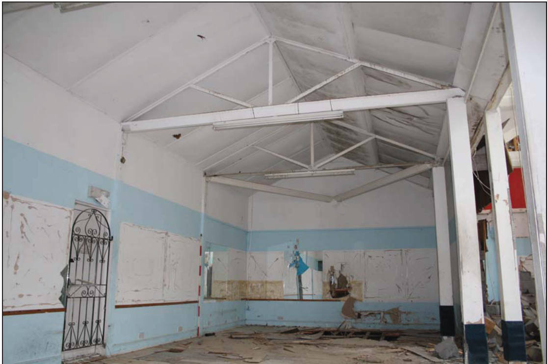
11 West side of Range 4 (Area 9) at upper level showing roof structure, taken from the east (24)
