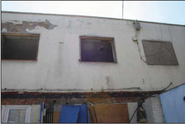
43 Upper level of the north façade of Range 1, taken from the north
