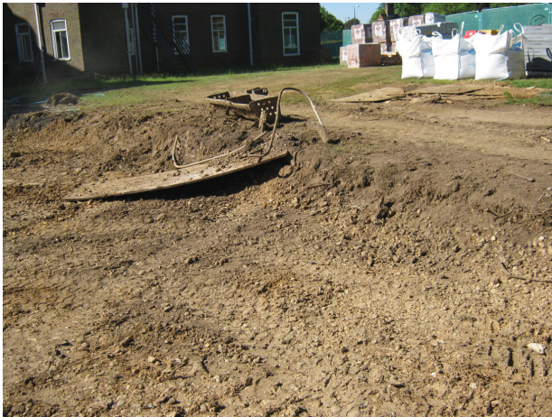
DP 3 General view of groundworks within footprint of proposed extension, looking south
