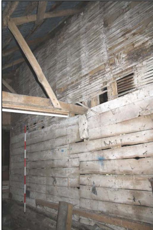
Plate 8 Upper laths and lower weather boarding, original external barn elevation seen in the outshut, taken from the north (DP 19)
