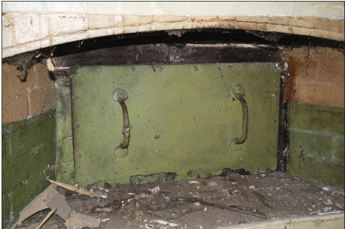
Plate 3 Door of the later inserted oven in the side of the Period B chimney stack of the rear kitchen, taken from the north-west (16)
