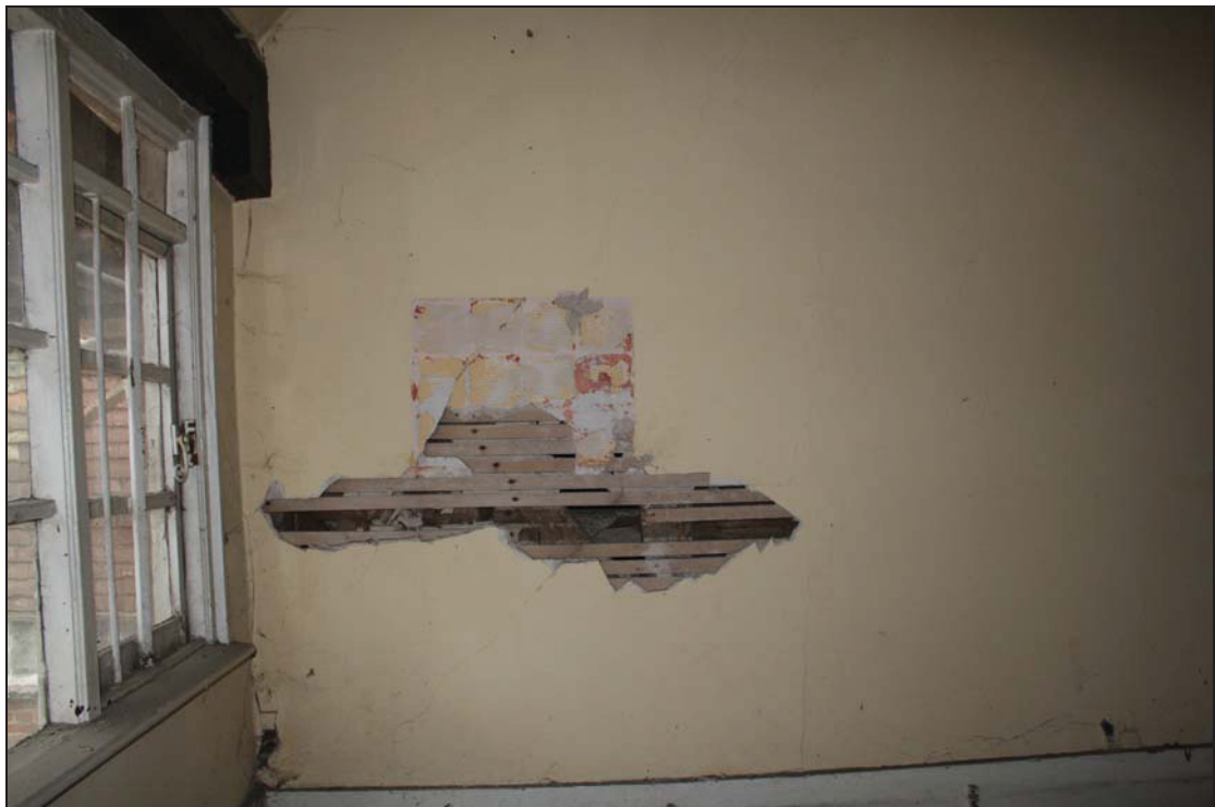
Plate 6 Section of plasterwork removed on the south wall of the second northern service chamber, taken from the north (30)
