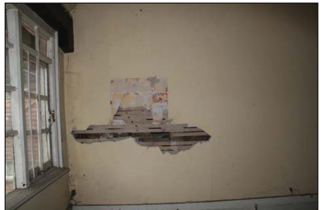
30 Section of plasterwork removed on the south wall of the second northern service chamber, taken from the north
