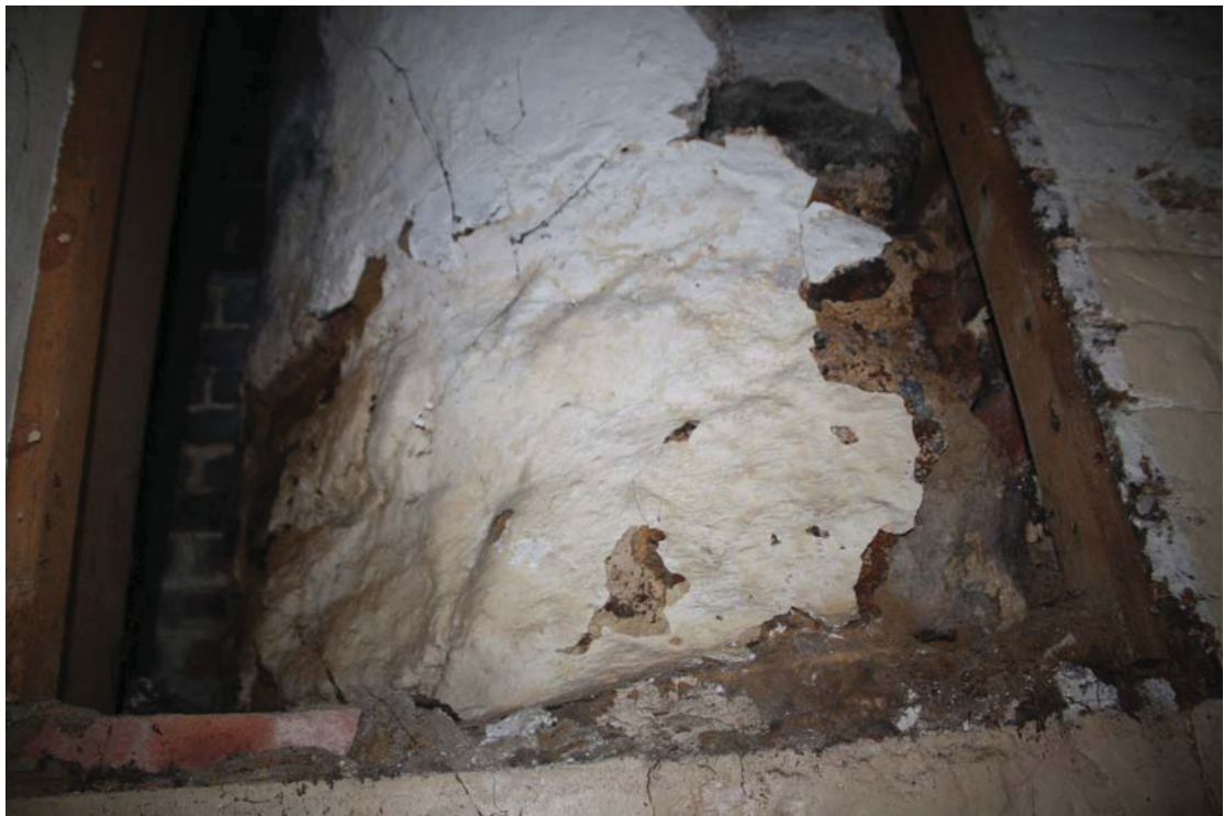
Plate 2 Detail showing the north side of the principal chimney stack, taken from the north (13)
