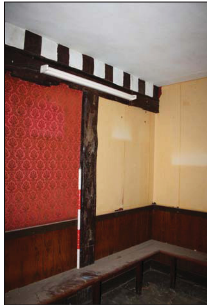
38 Formerly external wall of the main range parlour showing partially surviving timber-frame, taken from the north-west
