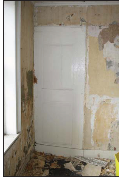
26 Fixed doorway in the south-corner of the new parlour chamber, taken from the north-east
