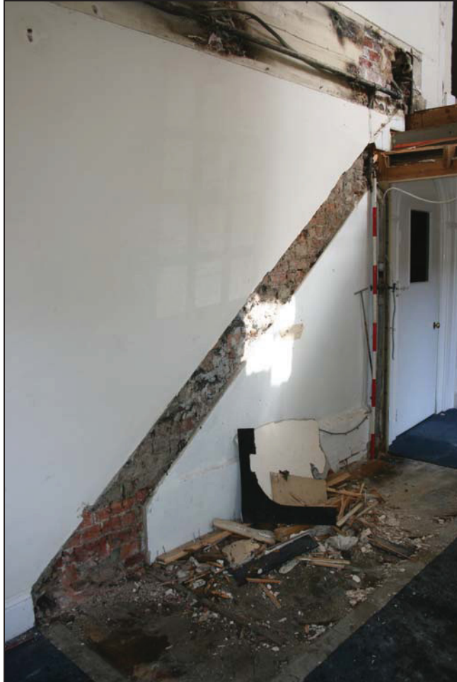
Plate 3 North-east side of the ground floor area showing exposed brickwork where staircase removed, taken from the west (3)
