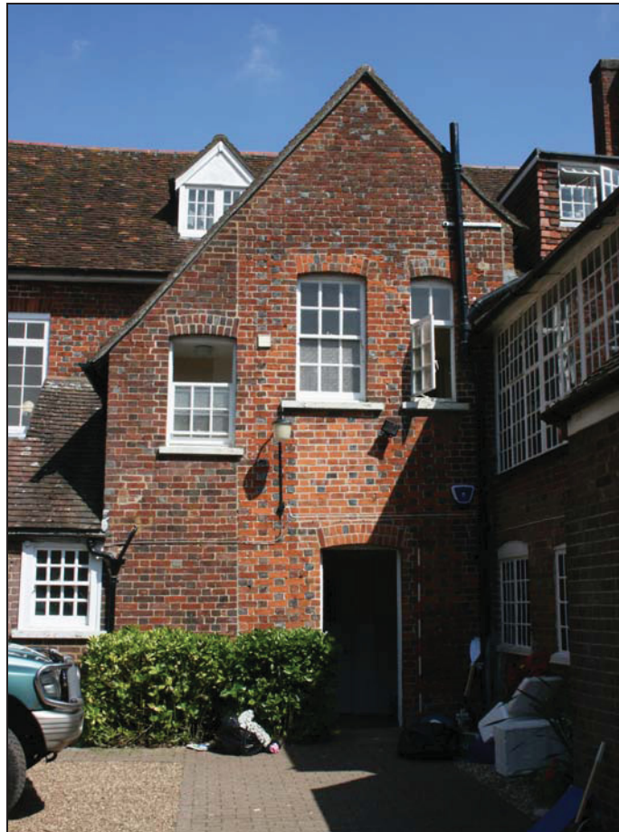
Plate 2 View of the stair turret on the south-west side of the main range of the house, taken from the south-west (2)
