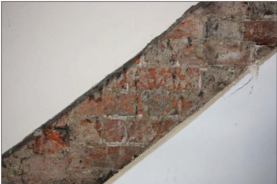
Plate 4 Detail of formerly external brickwork of the main range, taken from the south-west (5)
