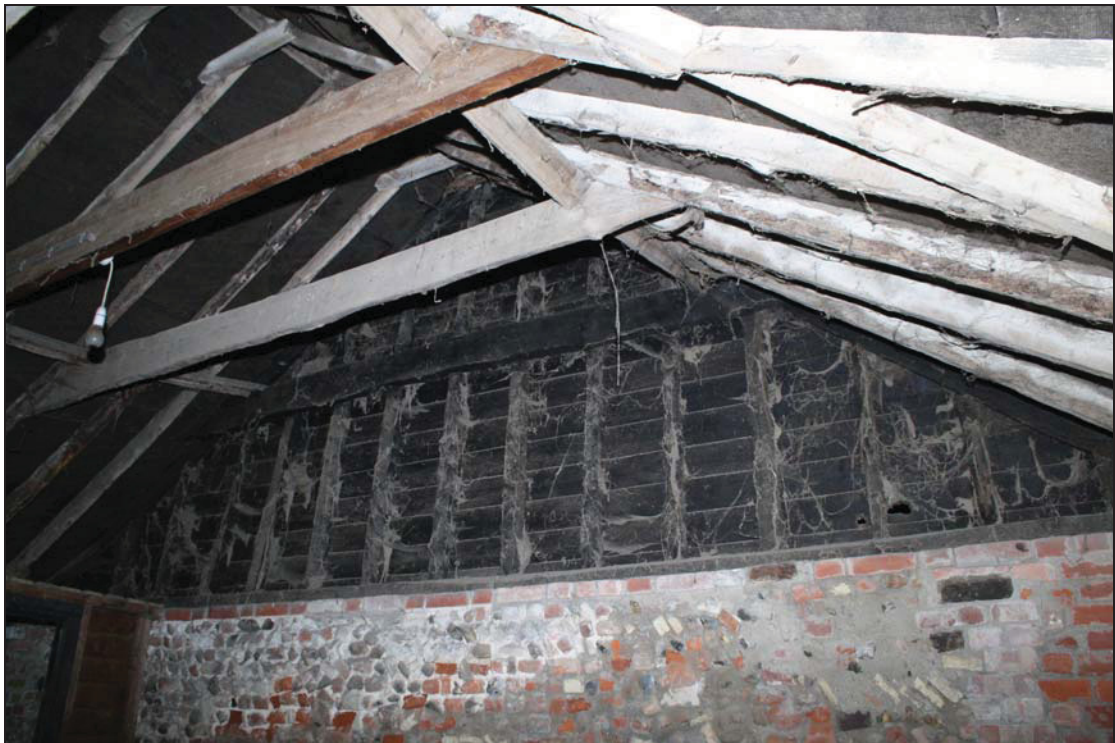
4 East wall of Bay 8 (partition between eastern and western elements), taken from the south (30)
