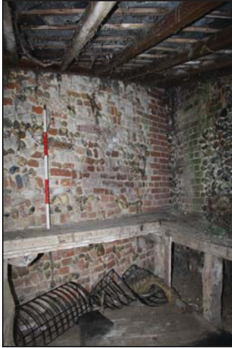
37 Interior of the small shed to the rear of the range, taken from the south-west
