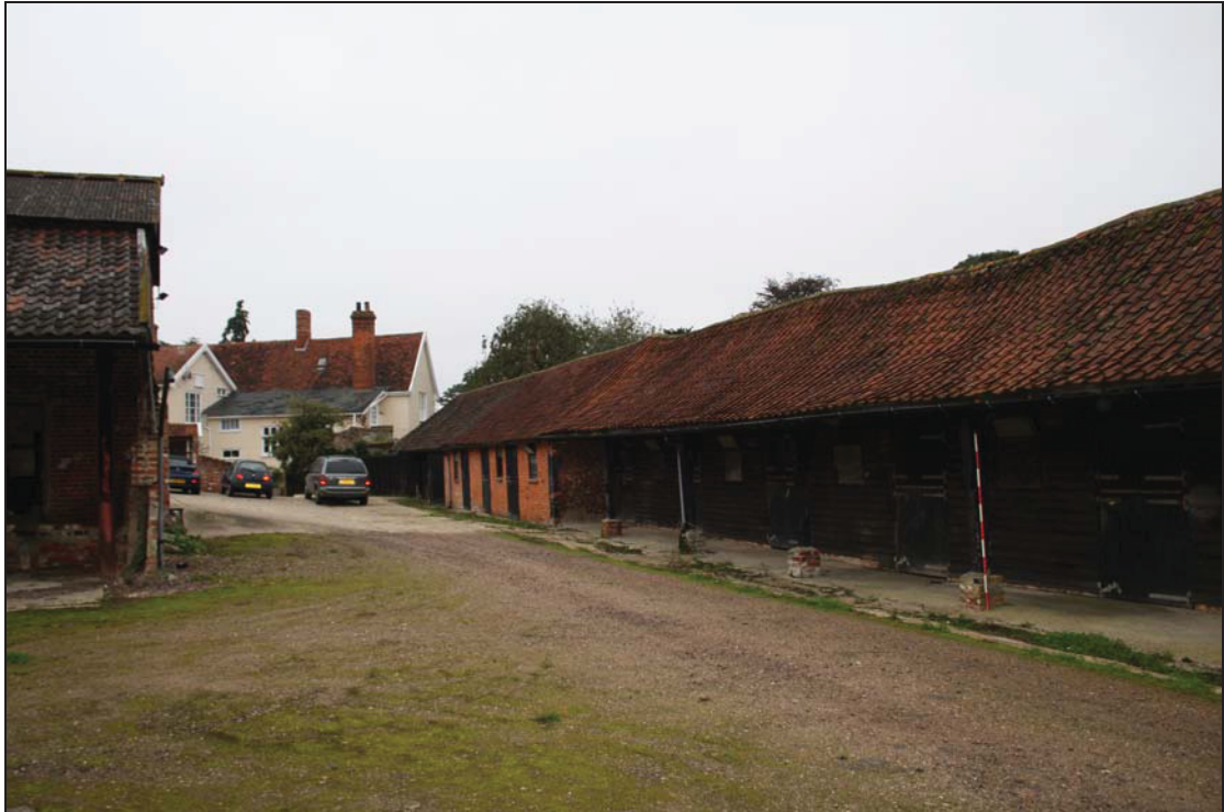
3 North elevation of the assessment range showing open-fronted area, taken from the west (03)
