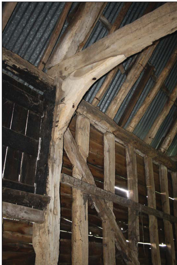
4 South-west end of the truss between Bays 3 and 4, taken from the east (37)
