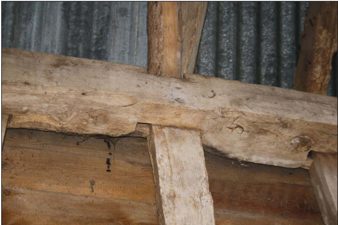
Plate 9 Unused configuration for a bay division on the north-east wall of Bay 1, taken from the west (26)
