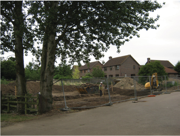
DP 1. Land to the east of Mill Lane, Kempston Mill, Kempston. View SE.
