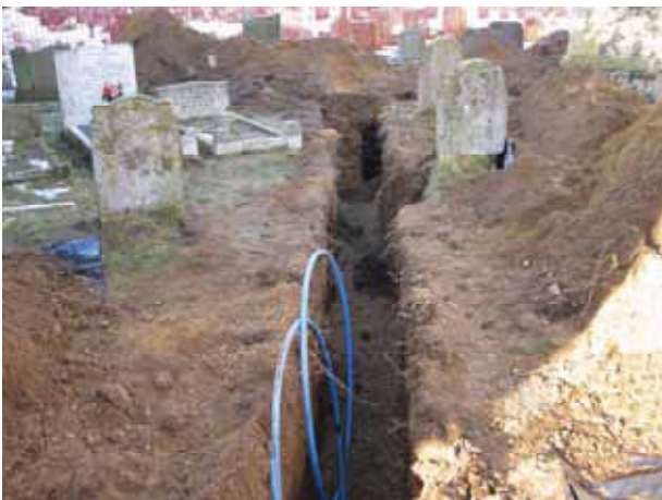
17 Post-excitation view of north-west to south-east trench run leading to the porch. Looking south-east.
