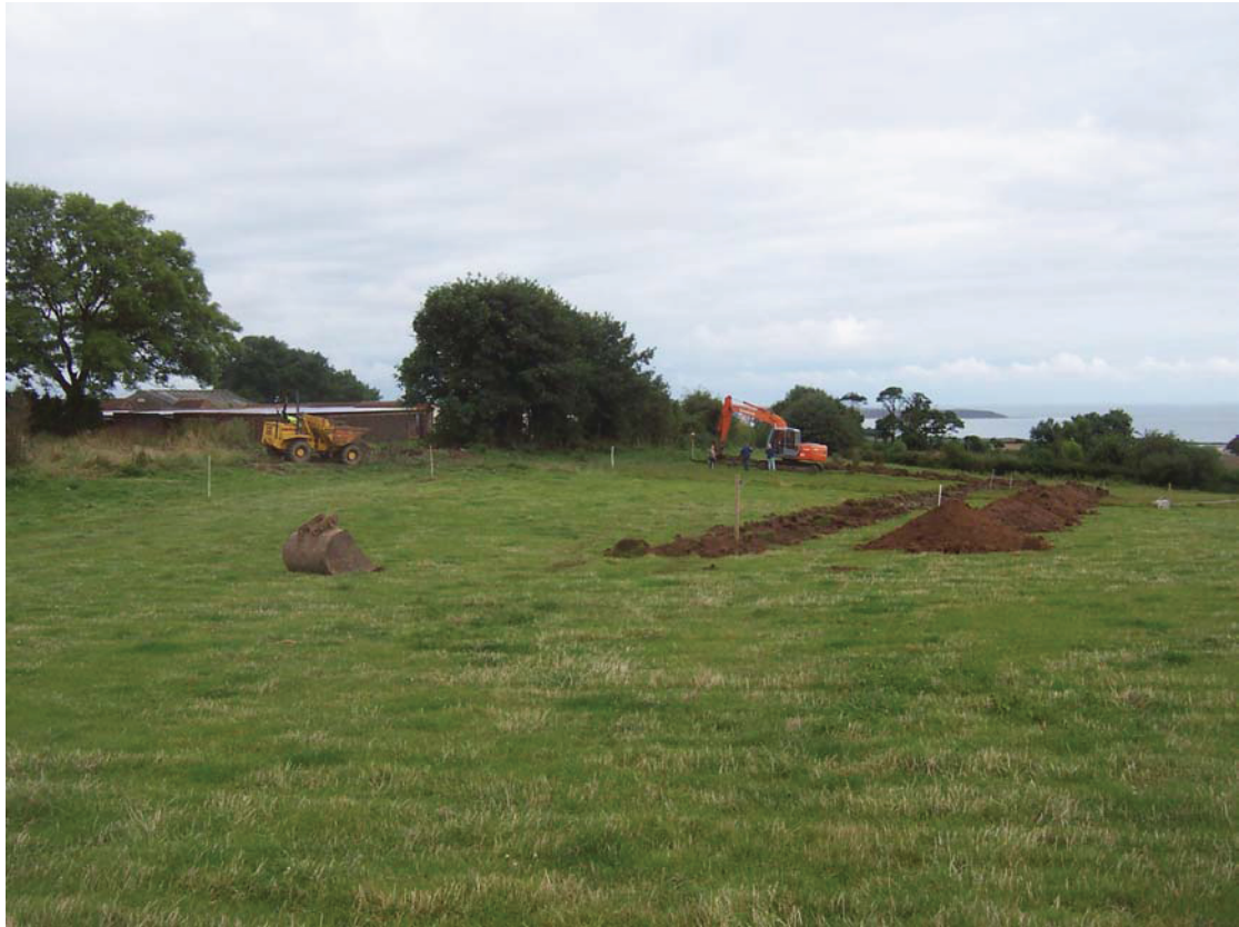
Plate 5 The L-shaped trench, the only groundworks on the site which involved the excavation of previously undisturbed soil, looking north-west.
