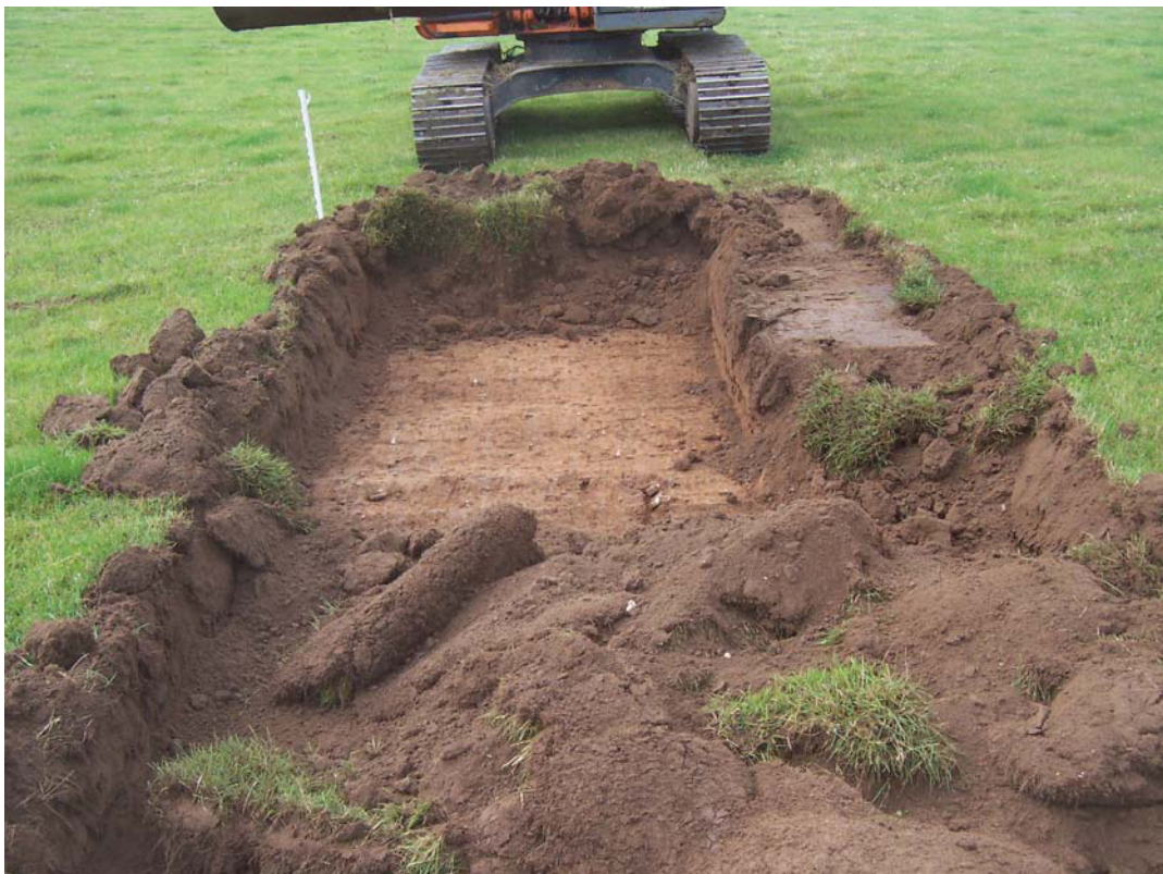
Plate 4 Cutting of the trench to obtain topsoil, note underlying sands (1002) looking east.
