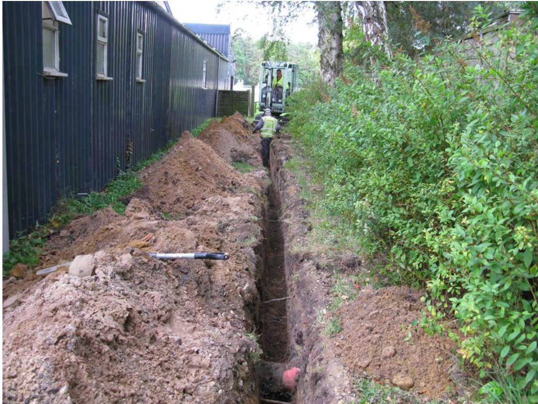
Plate 1 The northern east-west arm of trench 1 during excavations at the equestrian centre, viewed from the west.
