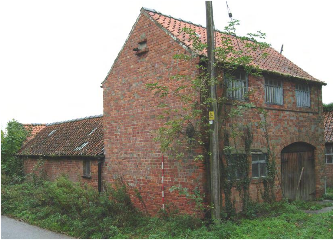
Plate 3 West elevation of building A, together with the south elevations of buildings A and B
