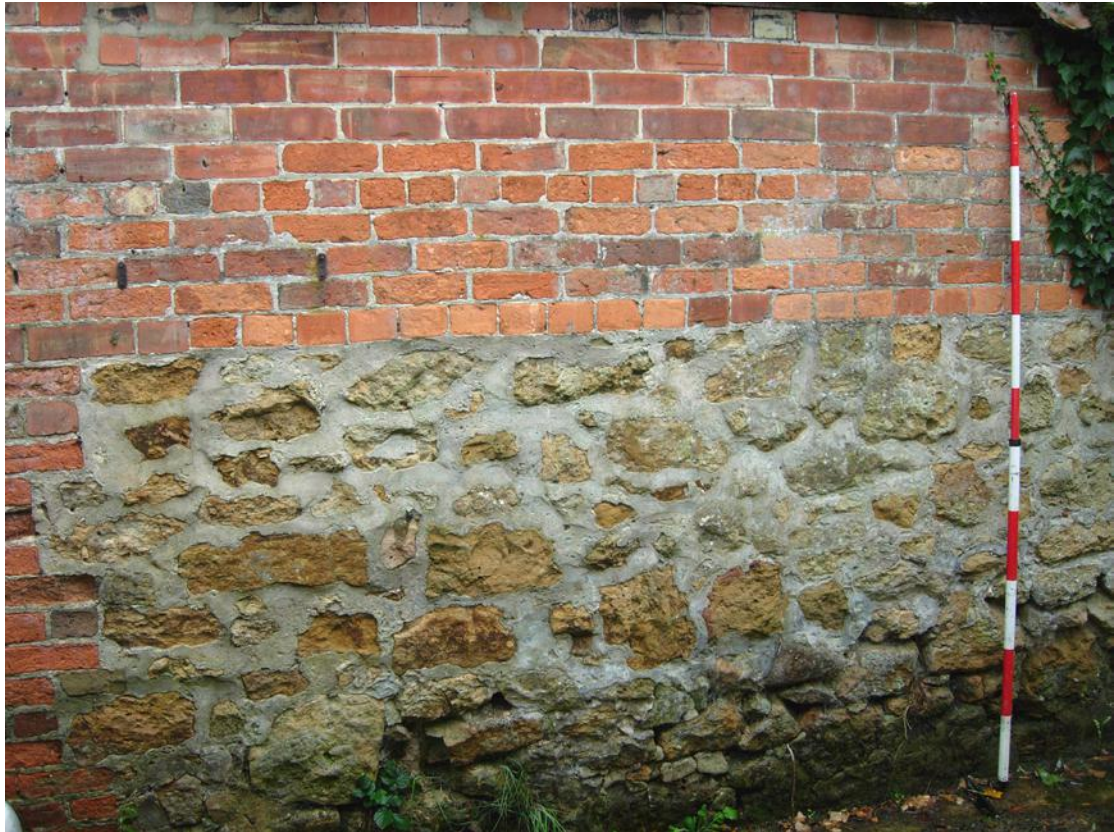
Plate 13 Rubble-stone walling in the western portion of the north elevation of building C
