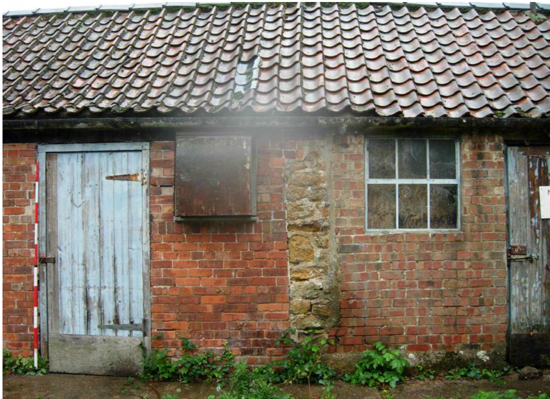
Plate 10 Detail of the south elevation of building C showing the end of a rubble-stone wall
