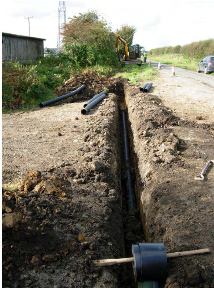
Plate 5 The middle section of the cable trench adjacent to Rigg Farm and looking west
