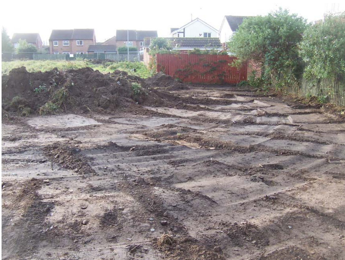
Plate 4 Stripping in the north-western area of the site, moving towards the south, looking from the north.
