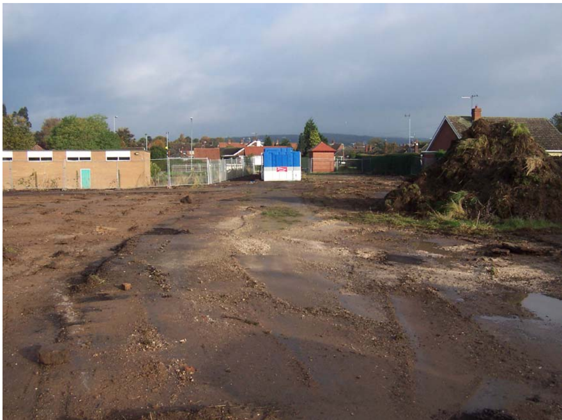
Plate 2 Stripping in the eastern and northern areas of the site, looking north.
