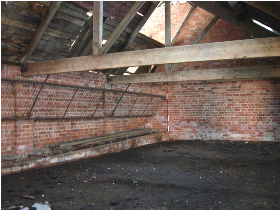
Plate 28 Low manger and hay rack along the south-central side of the crew yard (2m scale)
