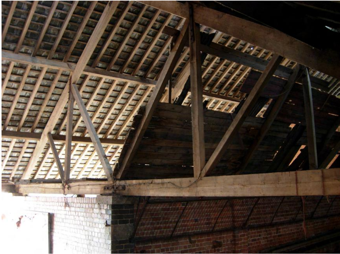
Plate 29 Queen-post and raking strut truss along the west side of the crew yard ramp
