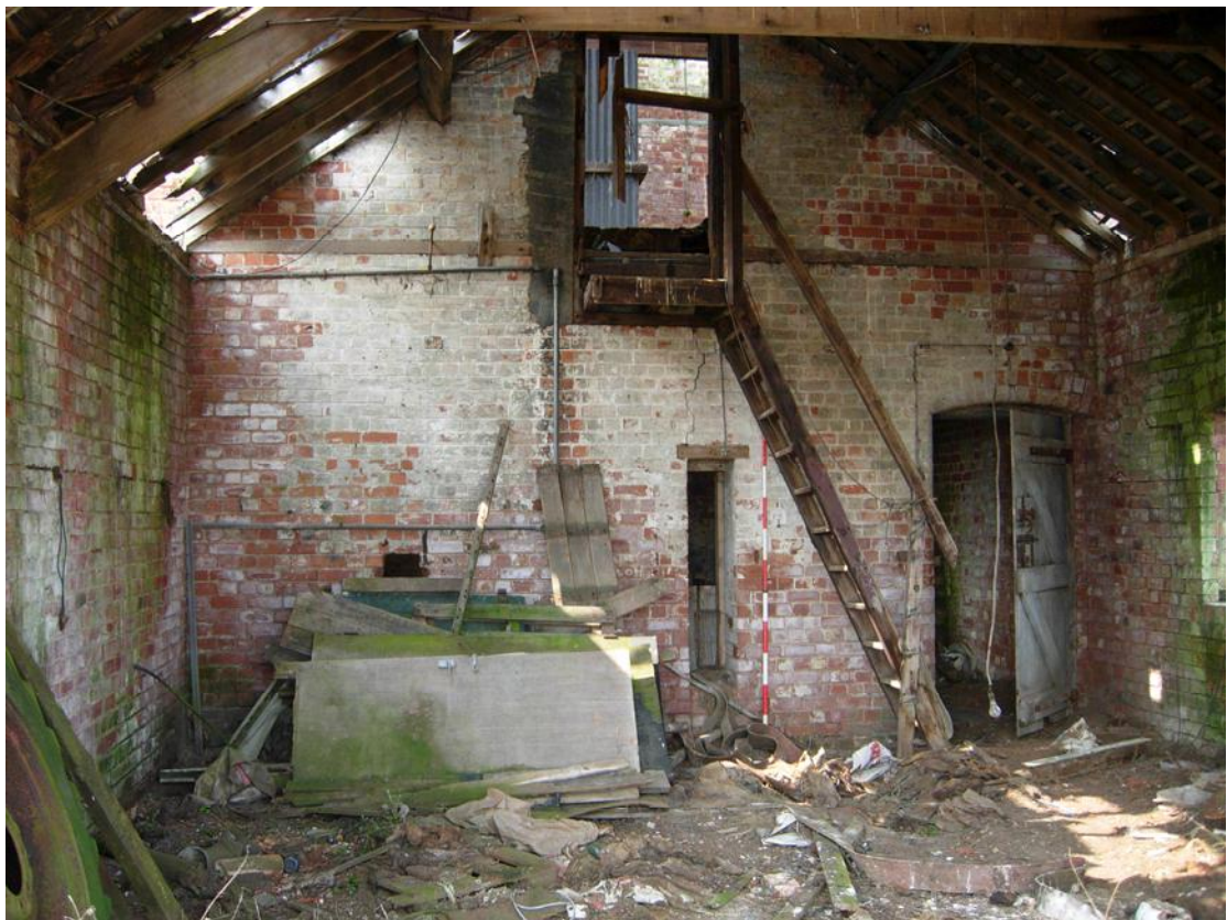
Plate 32 The engine house (room 11) viewed from the east (2m scale). Note the vertical transmission slot beneath the staircase
