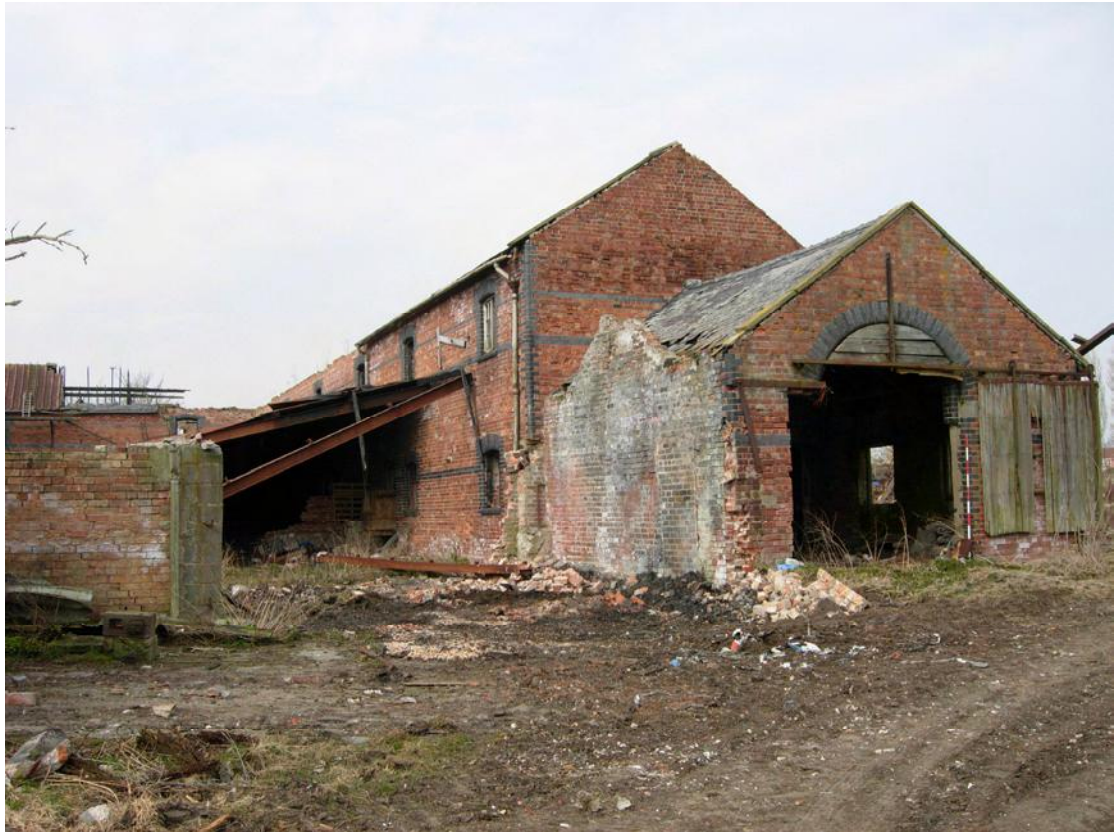
Plate 7 The engine house and north range viewed from the east (2m scale)
