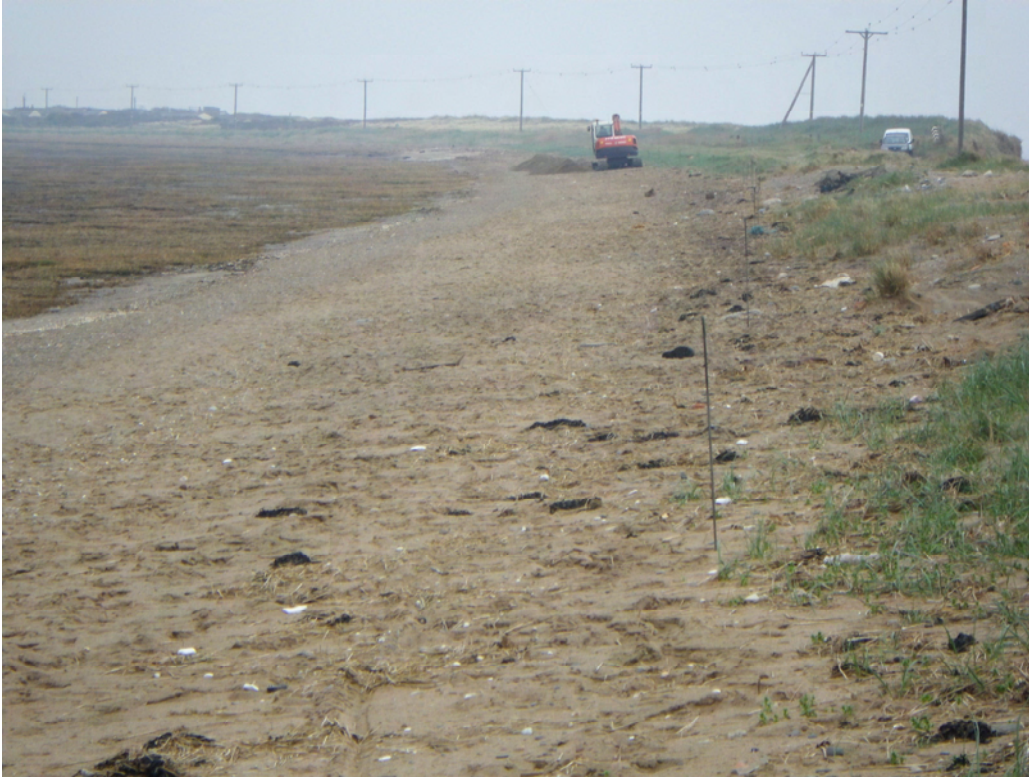
Plate 3 The site of the repositioned roadway along the western bank of Spurn peninsula. The metal road pins on the right demarcate the eastern side of the new road. Viewed from the south.
