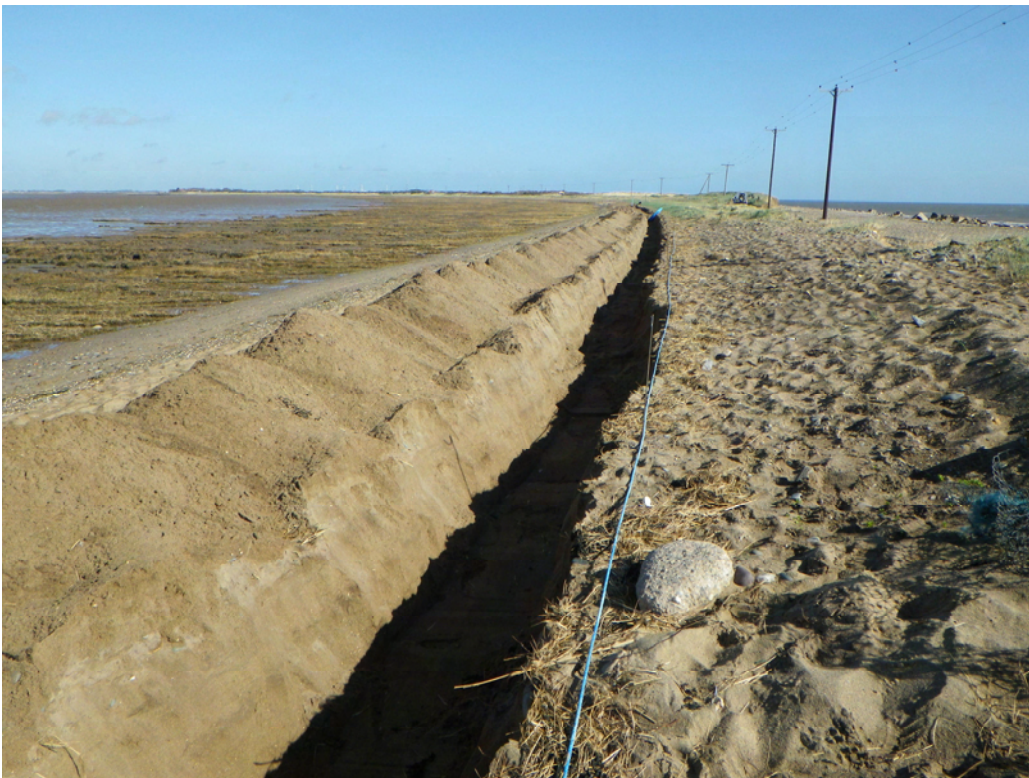
Plate 4 Showing the partially excavated water service pipe trench in the northern half of the proposed works. Viewed from the south.
