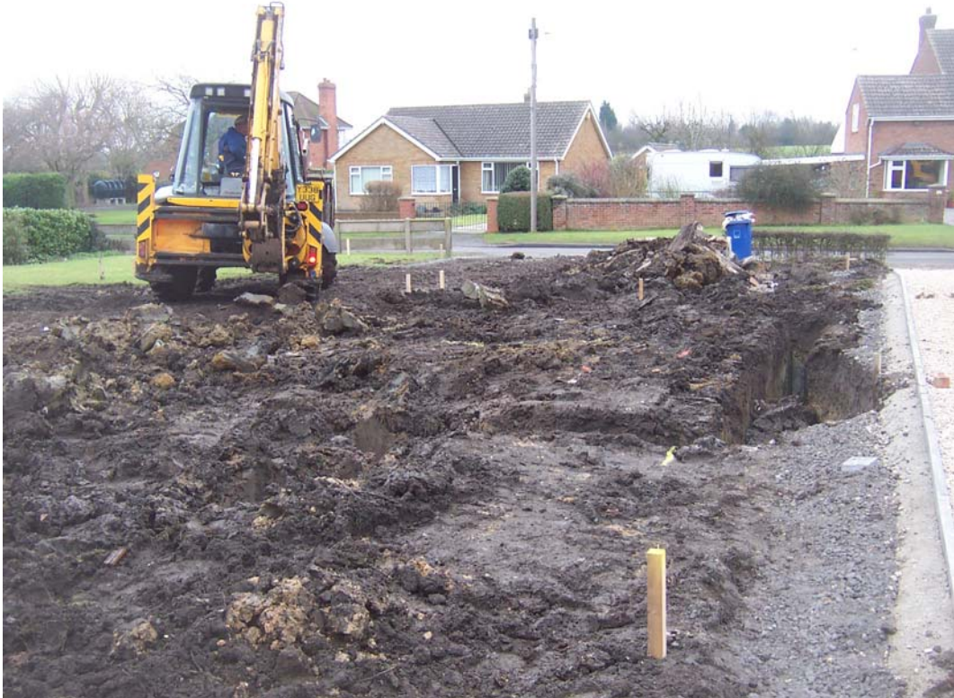
Plate 1 The site of the development during the excavation of the foundation trenches, looking southeast
