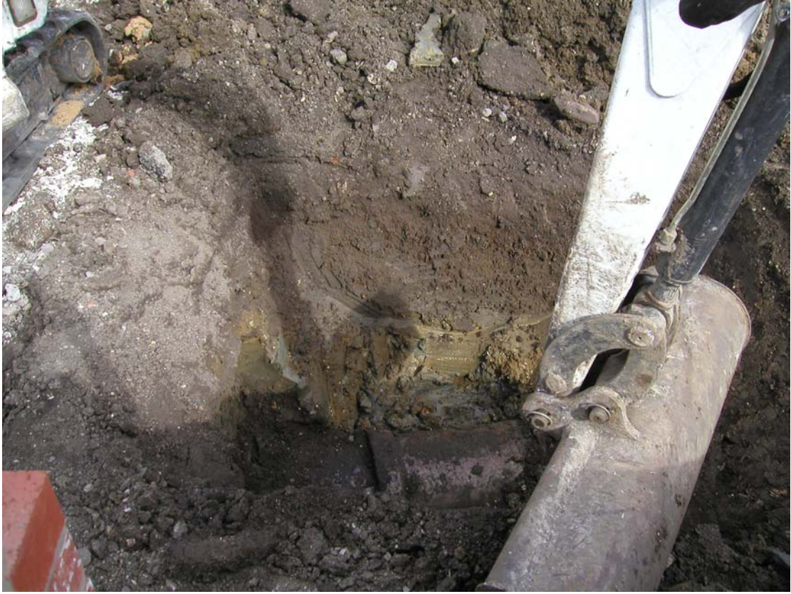
Plate 5 The excavation for the re-sited inspection chamber showing the large pipe in the base
