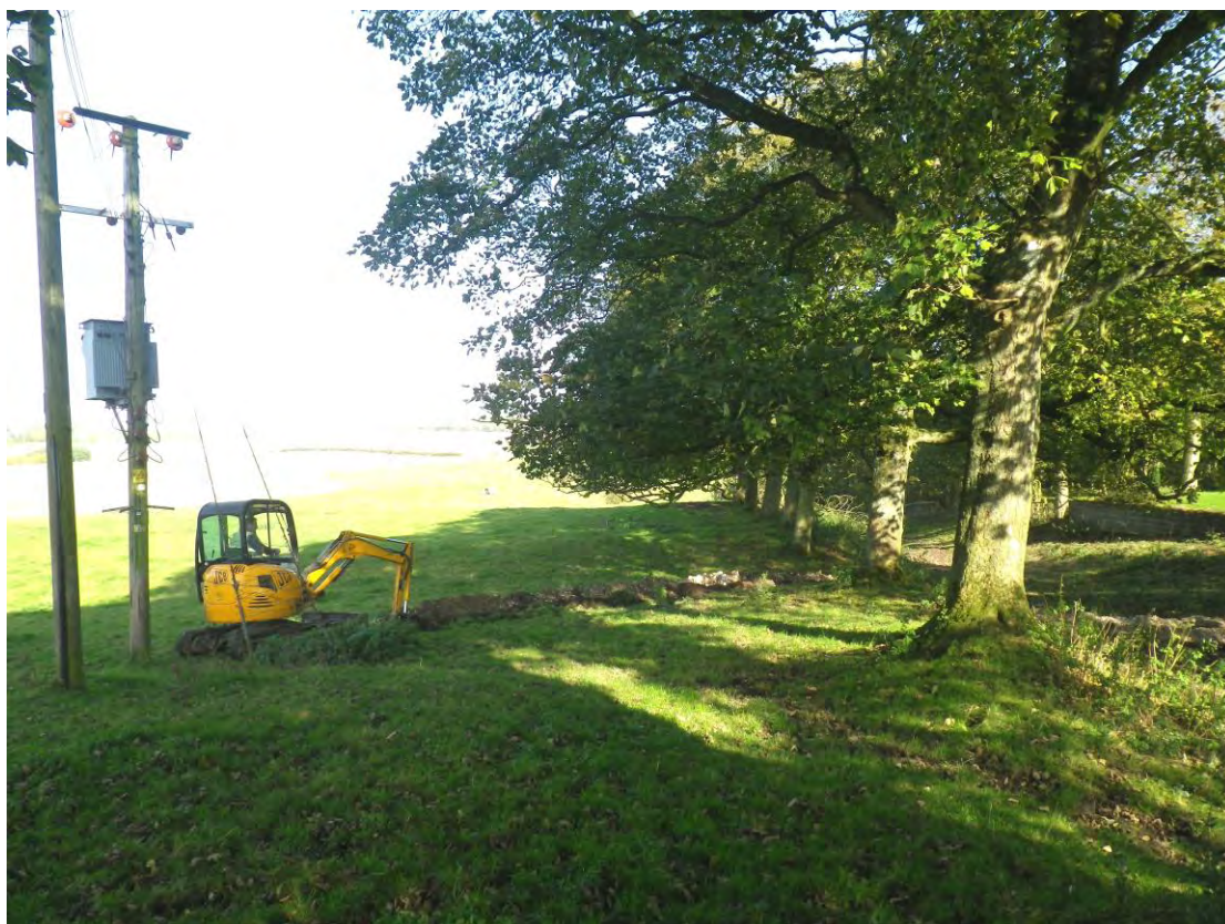
Plate 5 The trench within the DMV and nearing the transformer pole, viewed from the south
