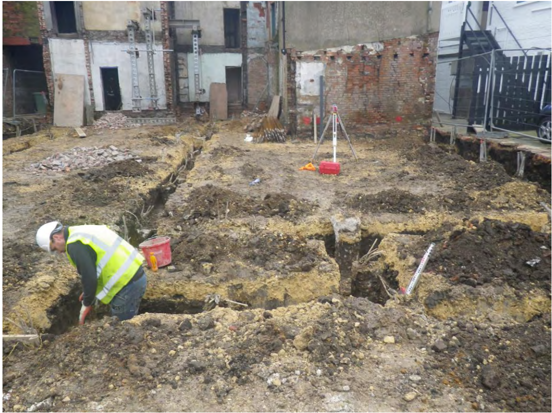
Plate 5 The beam slot foundations on the western side of the site, looking south
