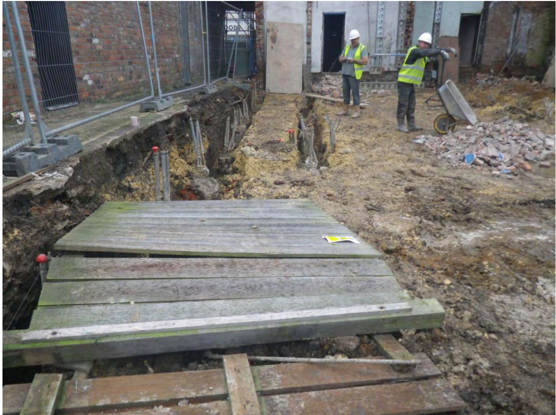
Plate 7 The eastern beam slot foundations with the stairwell to the rear of the image. Looking south
