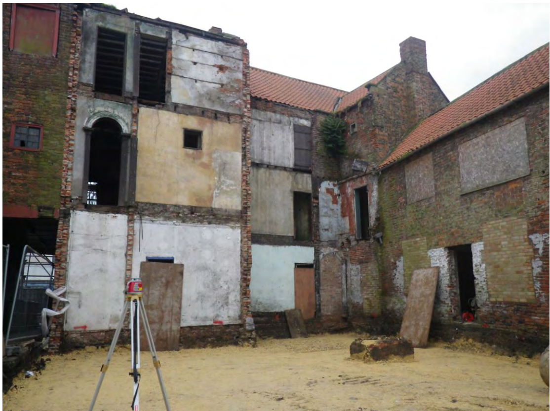
Plate 4 The stripped and stoned (1006) reduced level following the site strip, looking south-west
