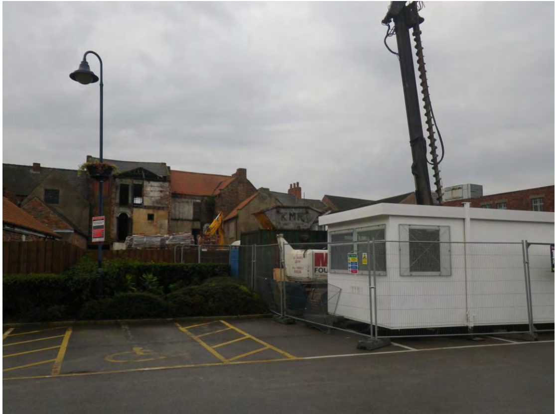
Plate 1 The site of the development from the rear of the properties, looking south-west
