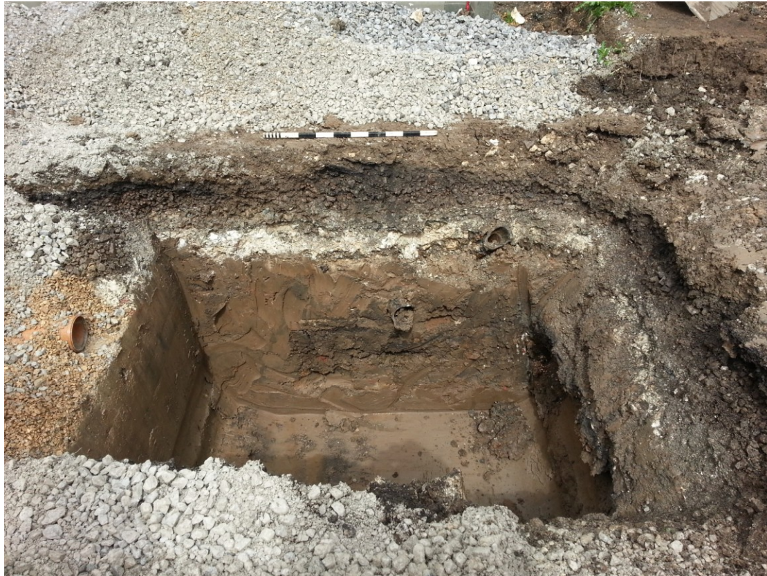
Plate 5 The completed excavation of the interceptor tank with rampart clay 110 in the base and slighted rampart remnants 109/108 and 105 above. Looking NW (1m scale)
