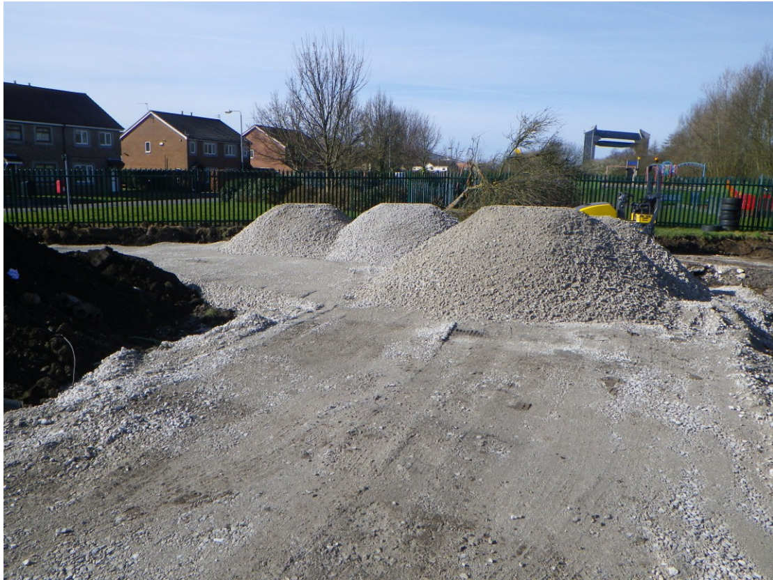
Plate 1 The reduced and stoned up central corridor of the new car parking area, looking SW
