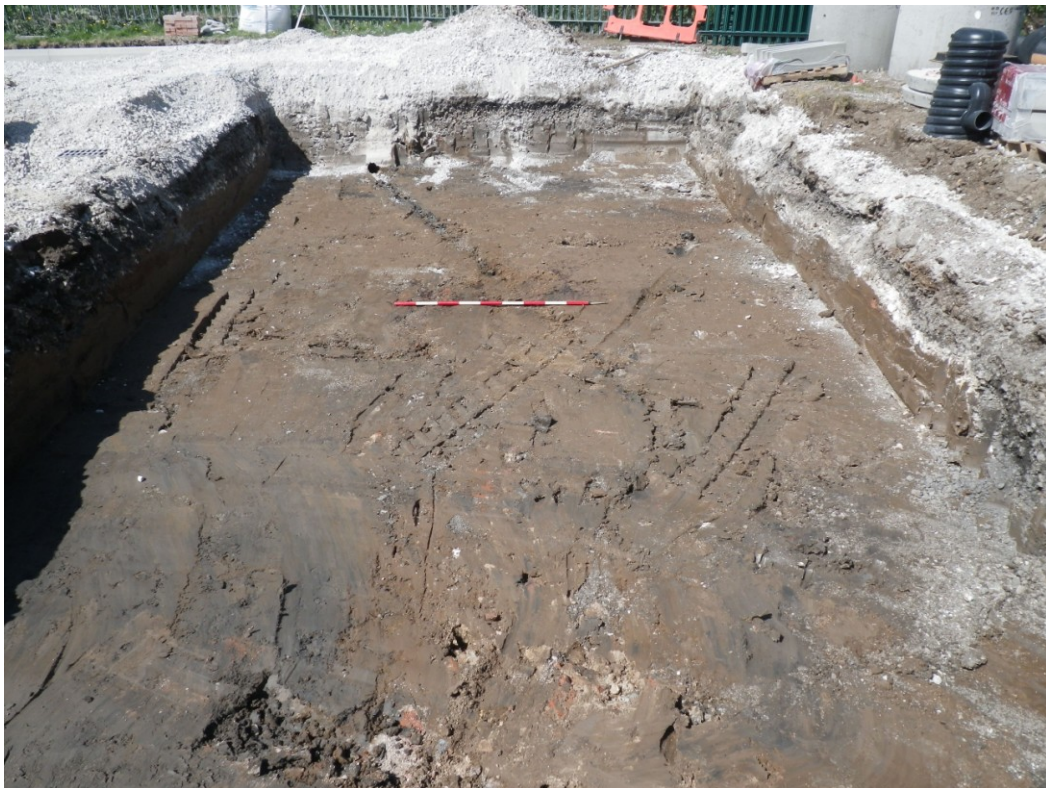
Plate 4 The completed excavation of the attenuation tank showing deposit 103 in the base, looking SW (2m scale)
