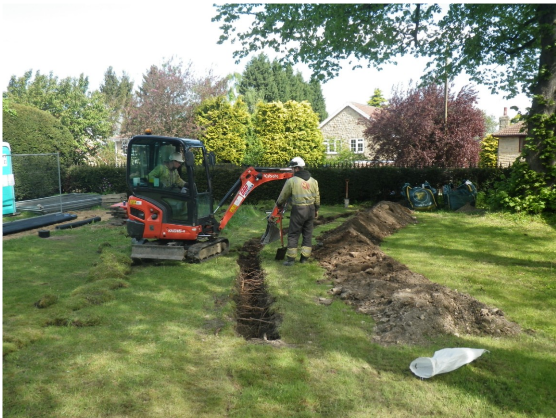
Plate 8 Showing excavation work at the northern end of the trench route (sections D and E), looking north
