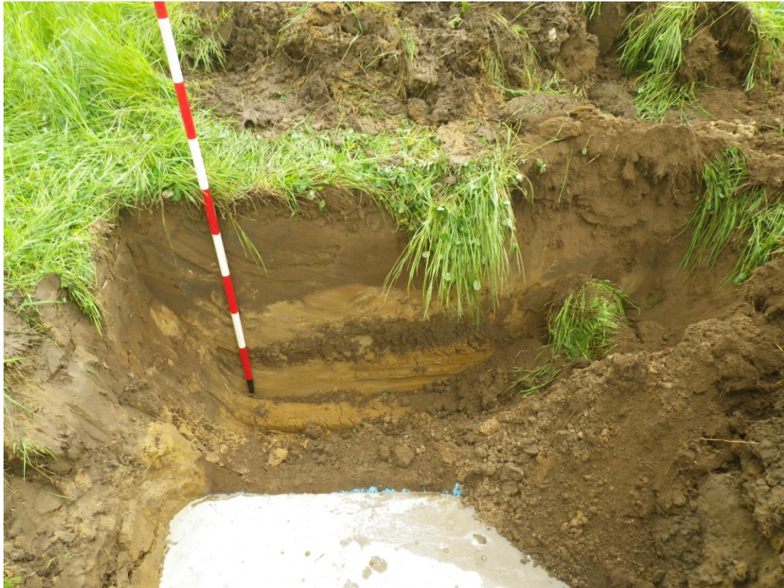
Plate 5 3m x 2m trench excavated at one of the field 2 pole holes to facilitate repair to damaged water pipe. Contexts 1001 and 1002 visible
