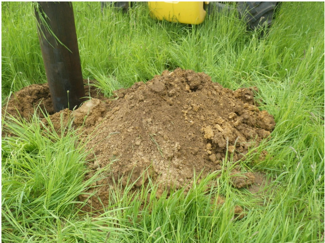
Plate 2 Typical spoil from pole hole (field 1) showing mix of topsoil (1001) and sand (1002)
