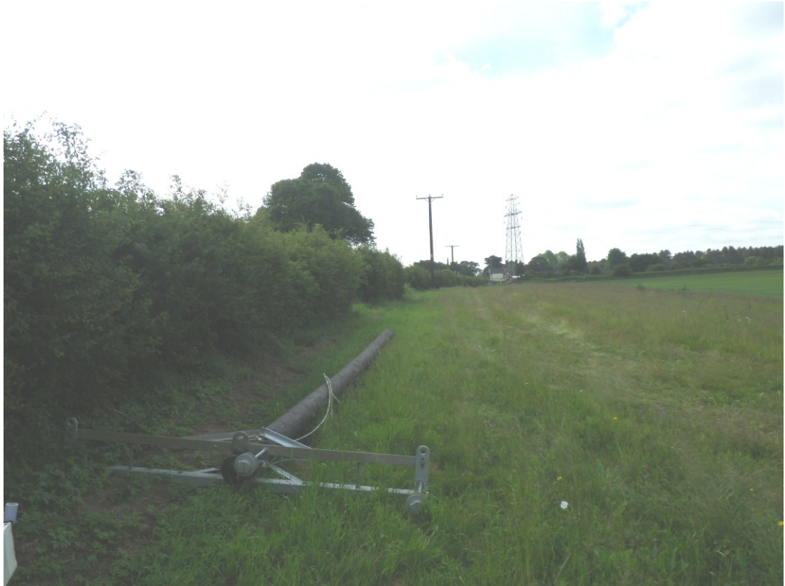
Plate 9 Pole replacement in progress along the eastern edge of field 4, viewed from the north
