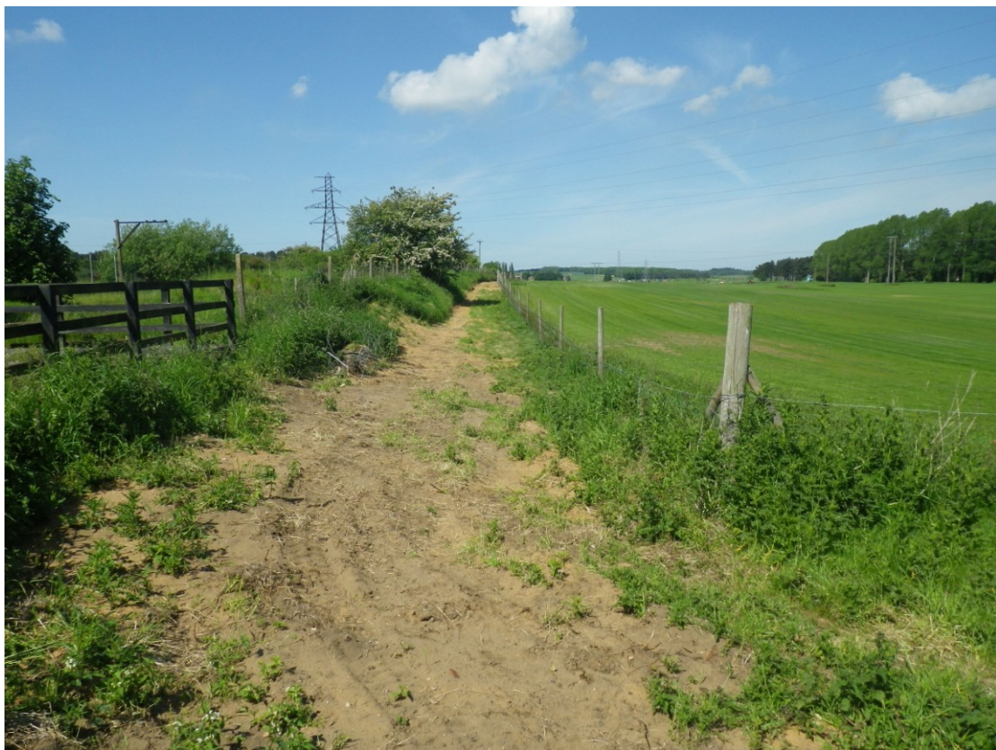
Plate 8 Back filled cable trench running along the south side of field 4, viewed from the east
