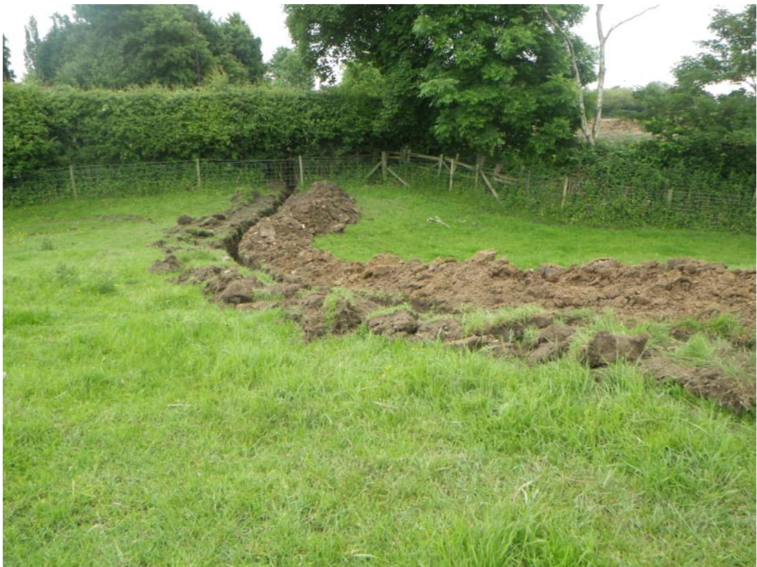
Plate 8 The cable trench as it passes down into the moat in the SW corner of the site to meet the site boundary, looking SW
