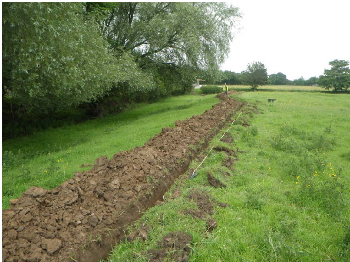
Plate 6 General view of the cable trench as it cuts along the upper western edge of the moat platform, looking NNW
