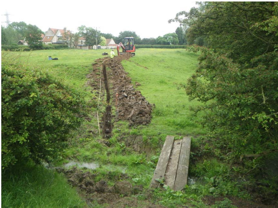
Plate 2 Initial cutting of the cable trench at the NW corner, starting in the moat working up onto the platform, looking SE
