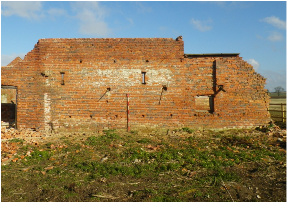
Plate 4 The eastern part of the south elevation of building 2, with the only extant part of building 1 to the right (2m scale)
