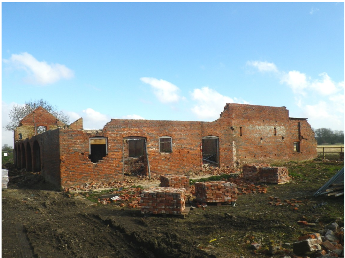
Plate 2 Buildings 2 and 3 viewed from the south-west across the site of the demolished building 1 (2m scale)
