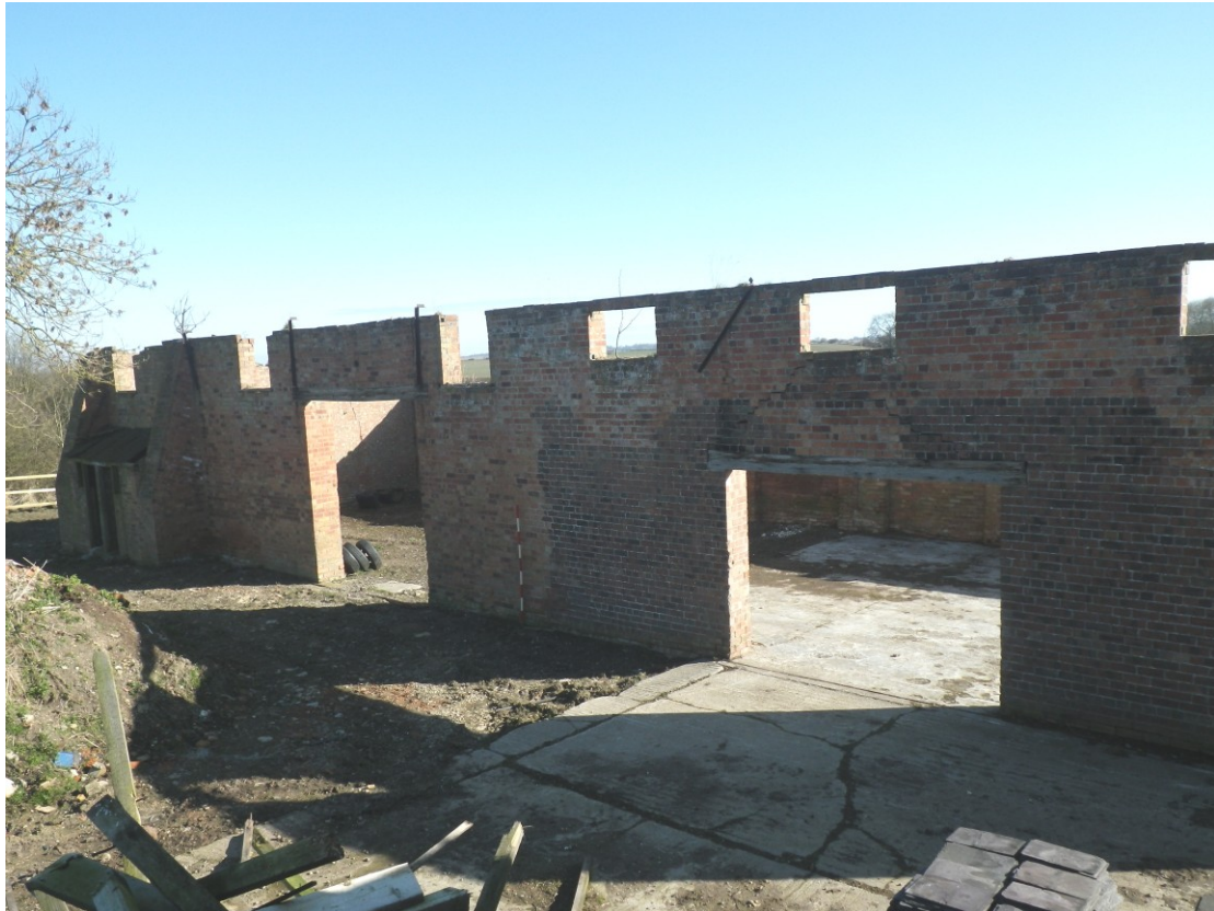
Plate 9 The west elevation of building 4 viewed from the top of the steps at the north end of building 3 (2m scale)
