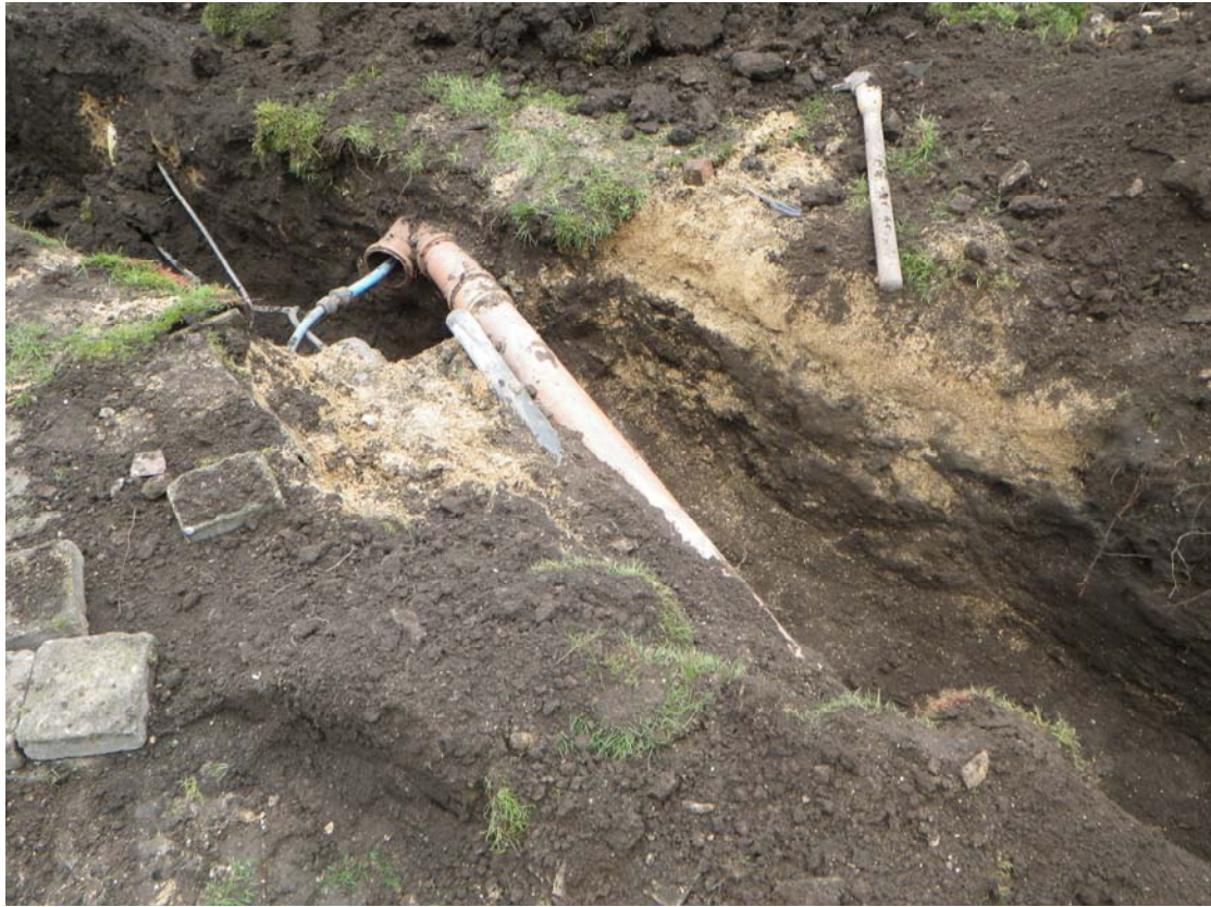
Plate 7 Significant modern service intrusions along the southern trench, looking NW.
