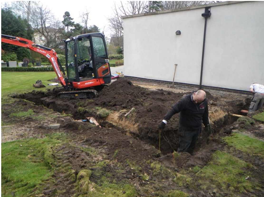
Plate 4 The foundation trenches for the new extension in their entirety, looking NW
