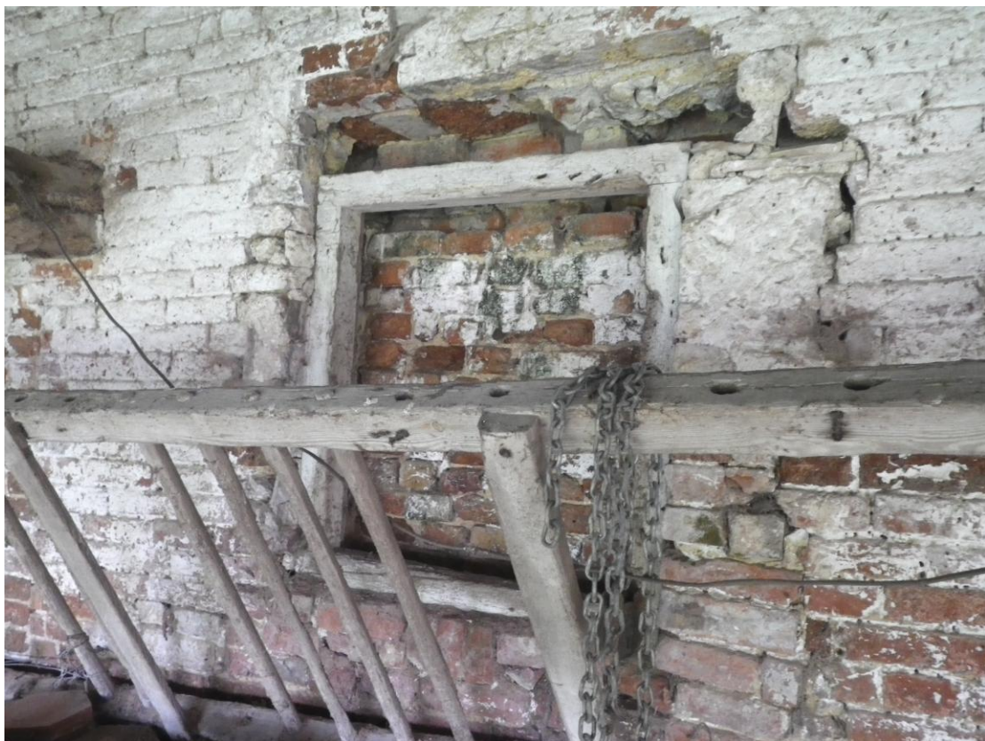
Plate 16 Partially blocked window (?) in the north wall with part of the manger in the foreground
