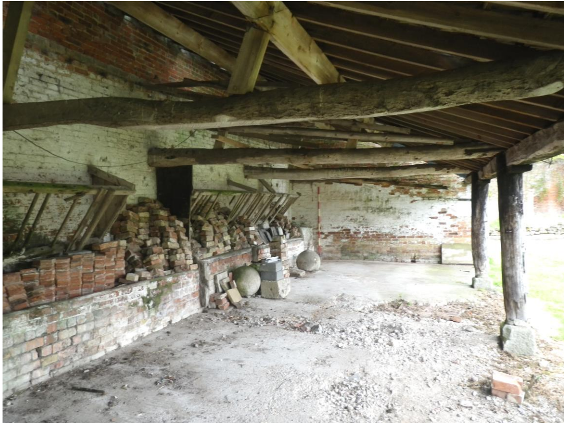
Plate 13 The interior of the eastern cart shed viewed from the south-west (2m scale)
