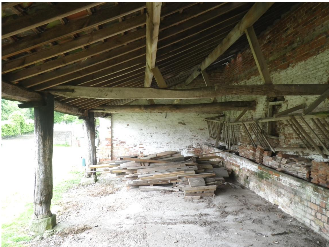
Plate 14 The interior of the eastern cart shed viewed from the north-east. Note the largely squared-off beam 3 in the foreground
