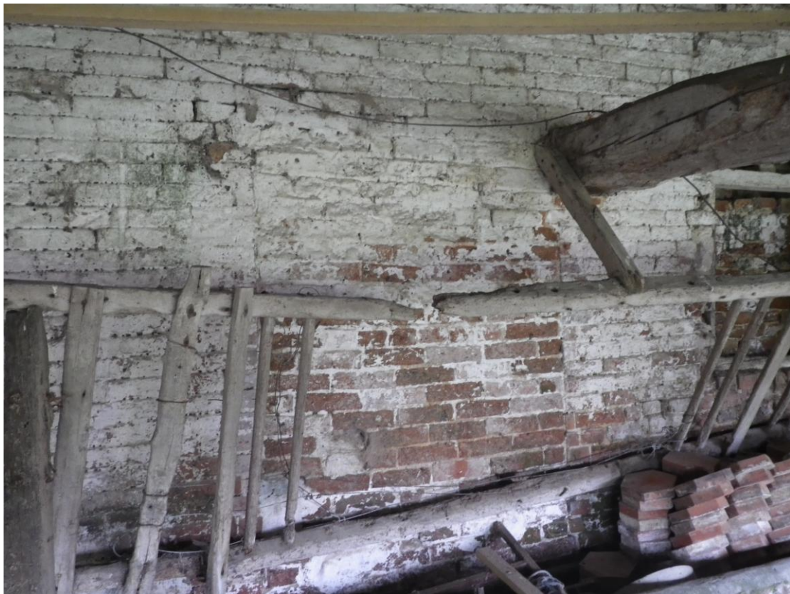
Plate 18 Straight joints in the north wall to the west of beam 4
