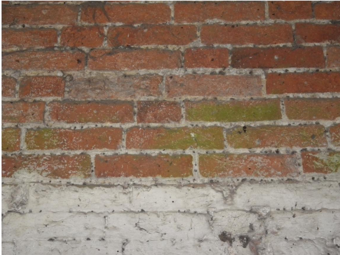
Plate 31 Damage to mortar caused by climbing plants in the north wall of the western cart shed
