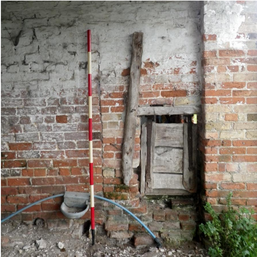
Plate 29 The wooden hatch viewed in room 3, here seen from the south-west (2m scale)
