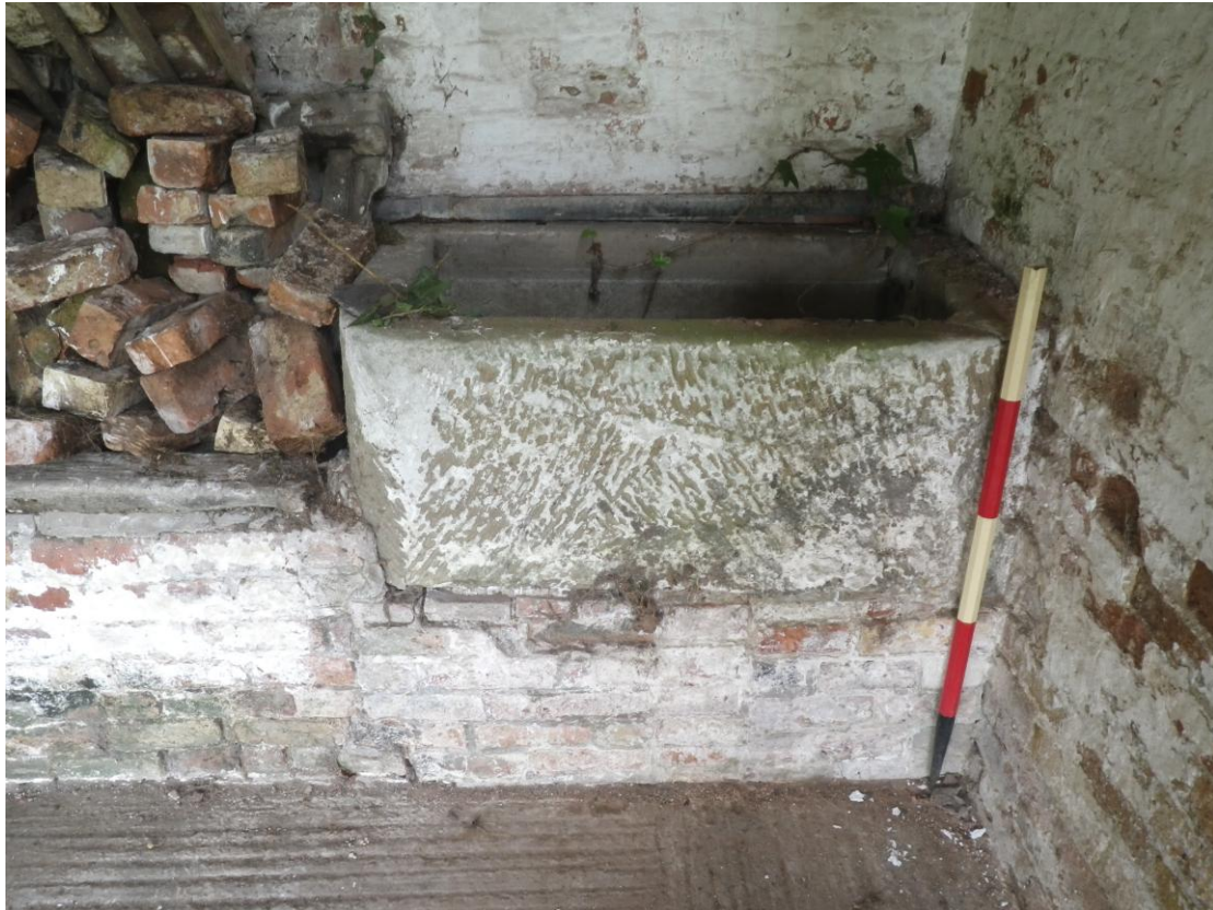
Plate 15 Stone trough at the east end of the feeding trough (1m scale)
