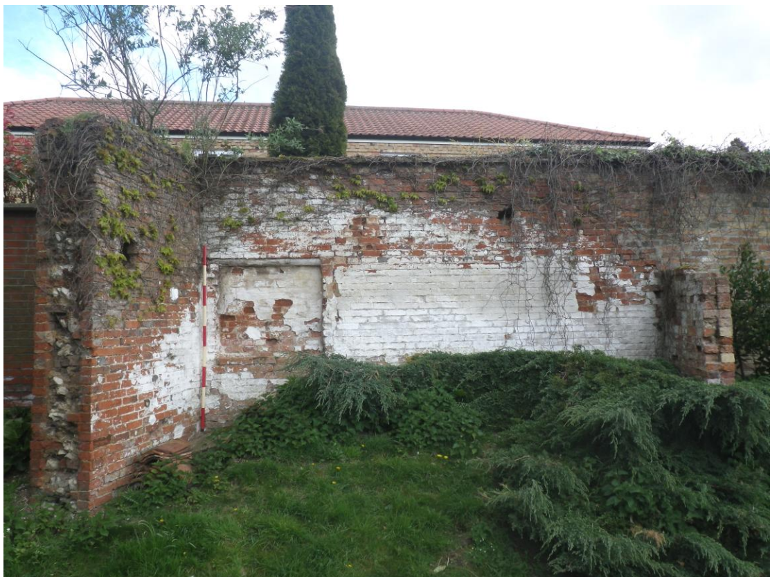
Plate 12 The former eastern end of the building, now detached from the rest of the building, as viewed from the south-west (2m scale)
