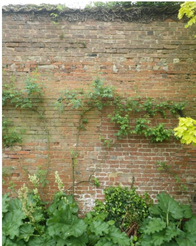
Plate 8 A portion of the southern part of the north elevation showing the change of brickwork in the lower portion and the raising of the wall height in the upper part
