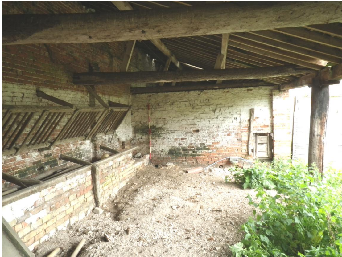
Plate 27 The interior of the western cart shed viewed from the south-west (2m scale)
