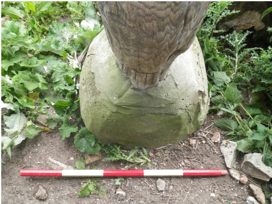
Plate 32 Concrete and cement base to the most easterly wooden post of the western cart shed (1m scale)
