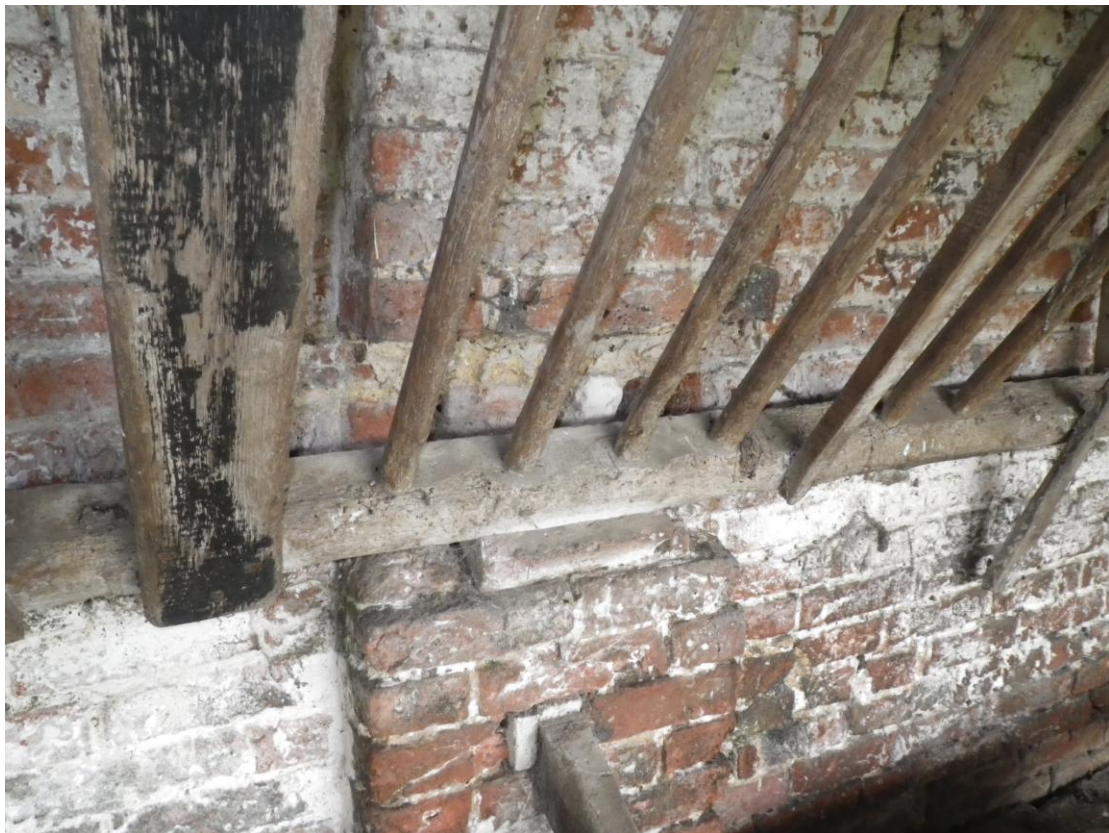
Plate 28 Detail of manger woodworking cutting into one of the buttresses of the north wall
