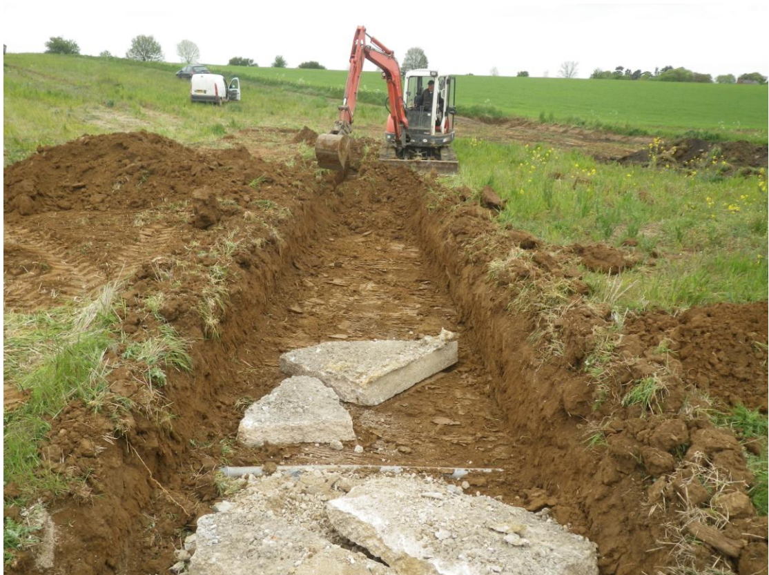
Plate 4: The trench excavated for the cinder track waste and other debris viewed from the south
