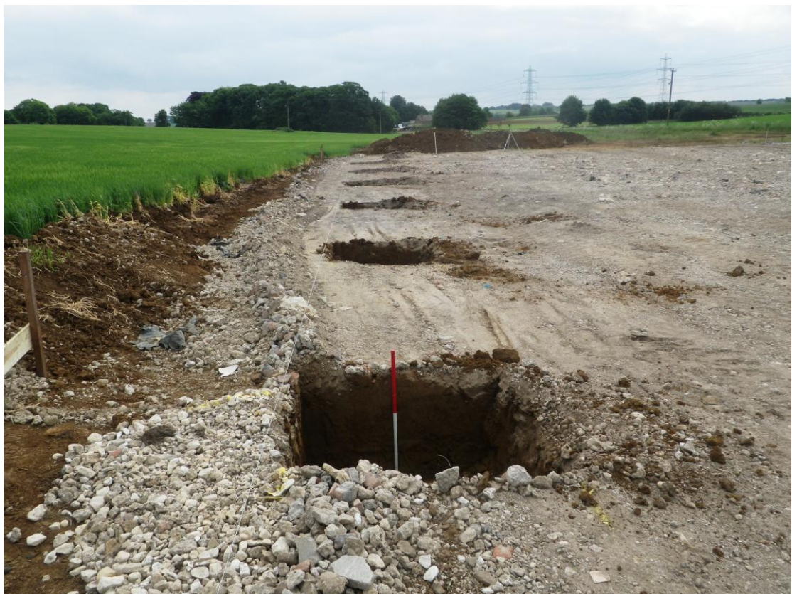
Plate 8: Foundation pits along the north side of the site, looking east (1m scale)
