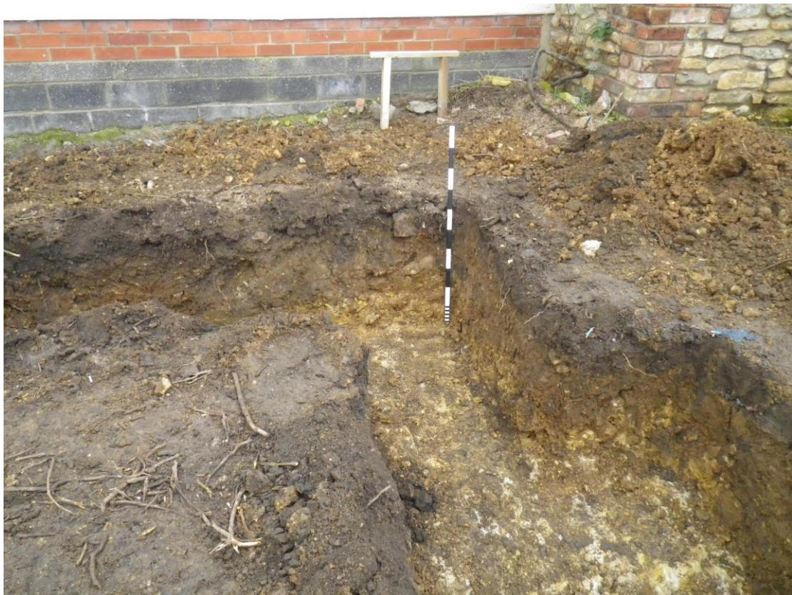
Plate 2 Shows the shallowness of subsoil layer 2 at the east of the foundations
