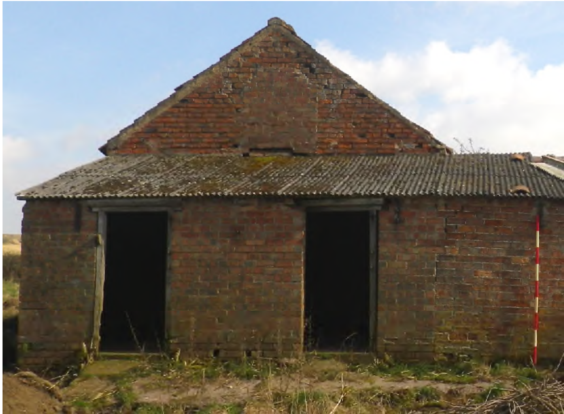
Plate 11 West facing elevation of Room 5 and the gable of Room 1 (2m scale)
