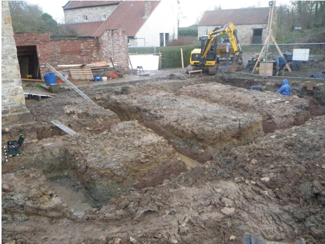
Plate 35 General view of the strip foundation trenches to the west and south of the mill, looking south-east
