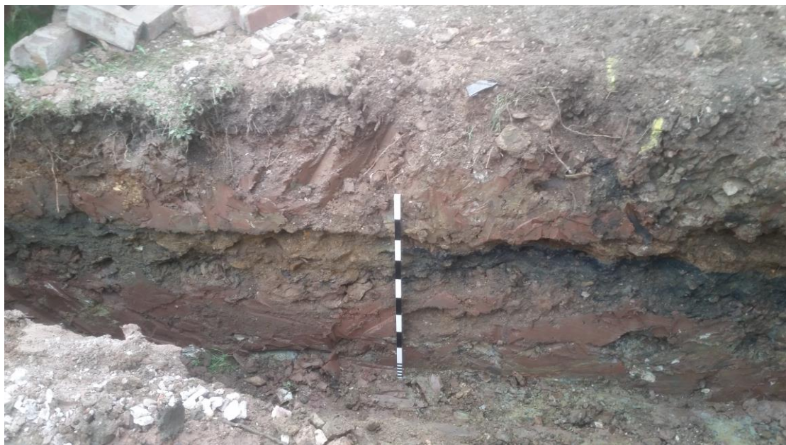
Plate 21 View of the levelling deposits to the south of the mill in the east foundations for the new build. Looking west, 1m scale
