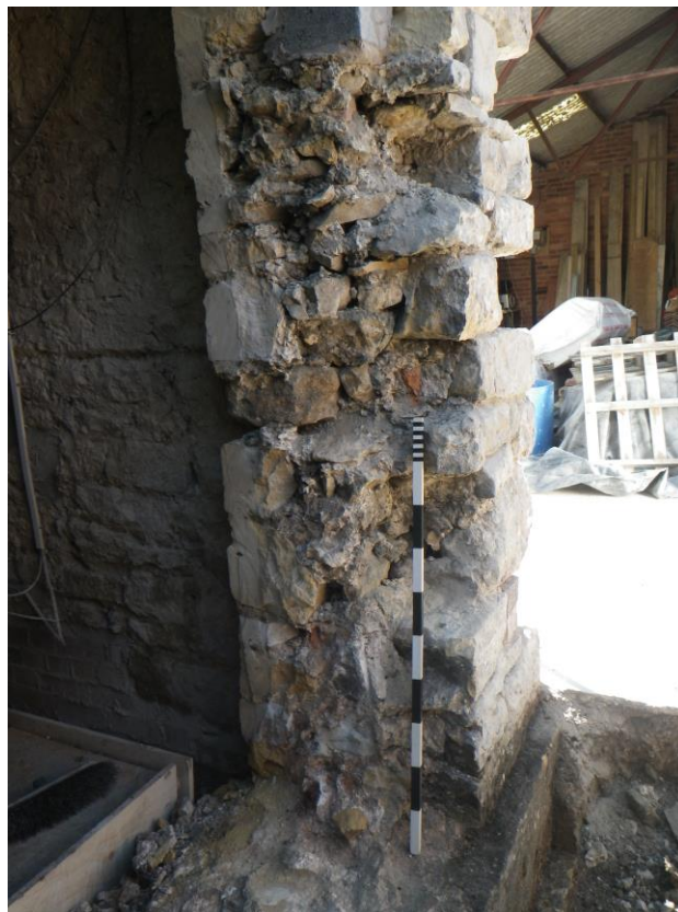
Plate 25 Cross section through the east side of the west mill wall (facing stones and rubble core), looking south, 1m scale
