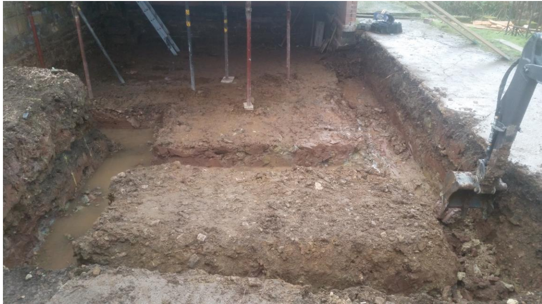
Plate 20 The reduced ground level and strip foundations for the work to the east side of the mill, looking north
