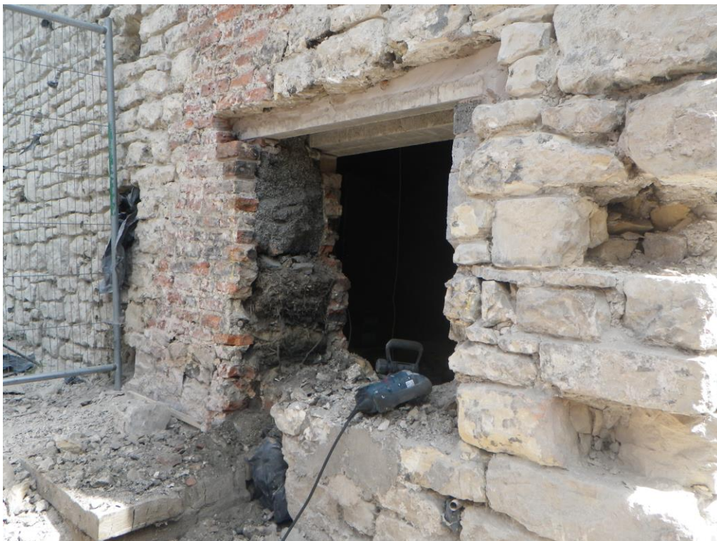
Plate 23 The cutting of the new doorway into the west side of the mill, bisecting the fireplace, looking north-east
