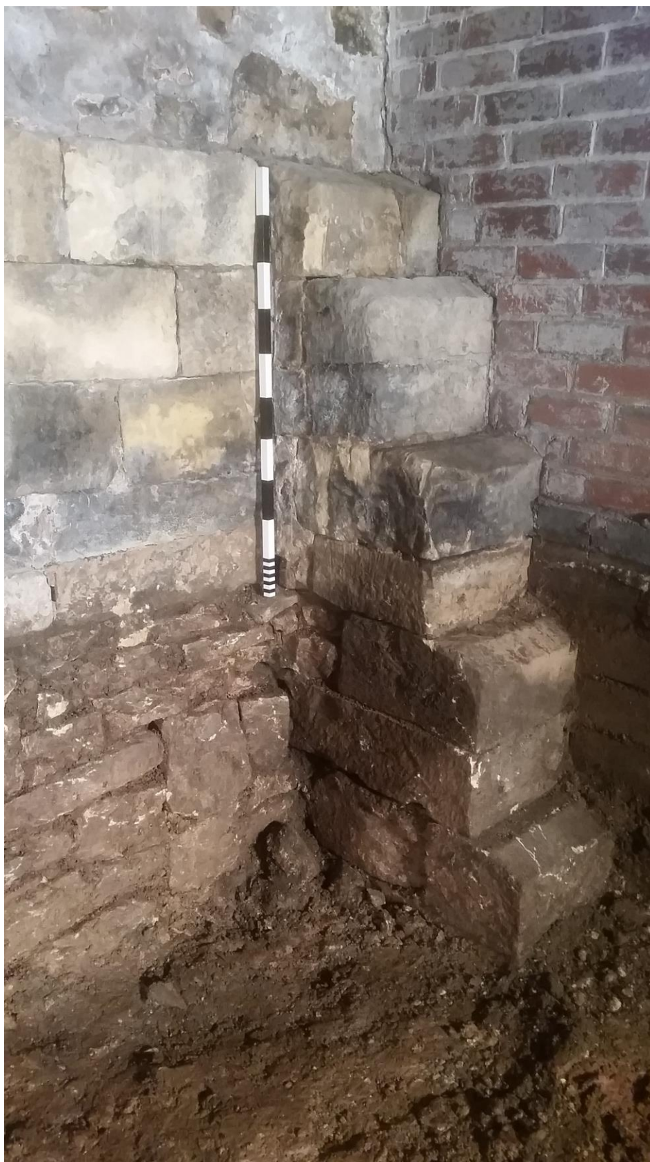
Plate 19 Detail view of the rebuilt footing 107 and rebuilt buttress 108 on the exterior north-east corner of the earlier mill wall foundations 105. Looking north-west, 1m scale
