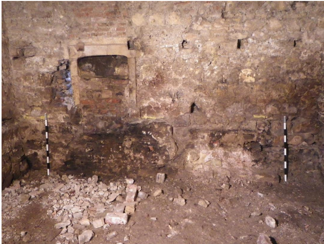
Plate 11 Full level ground reduction in the interior of the mill, showing fireplace 112 in the west wall and subsequent floor joist insertions. Looking west, 1m scales
