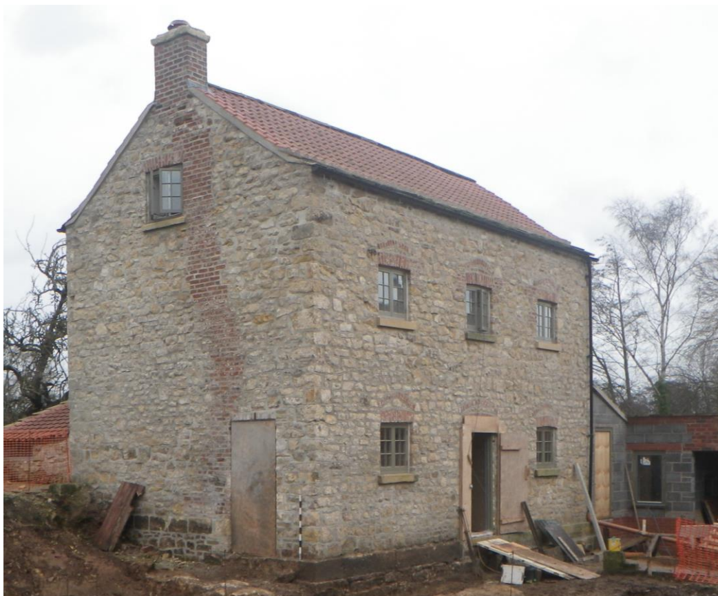
Plate 38 The south and west elevations of the mill after the removal of the render, looking north-east. 1m scale
