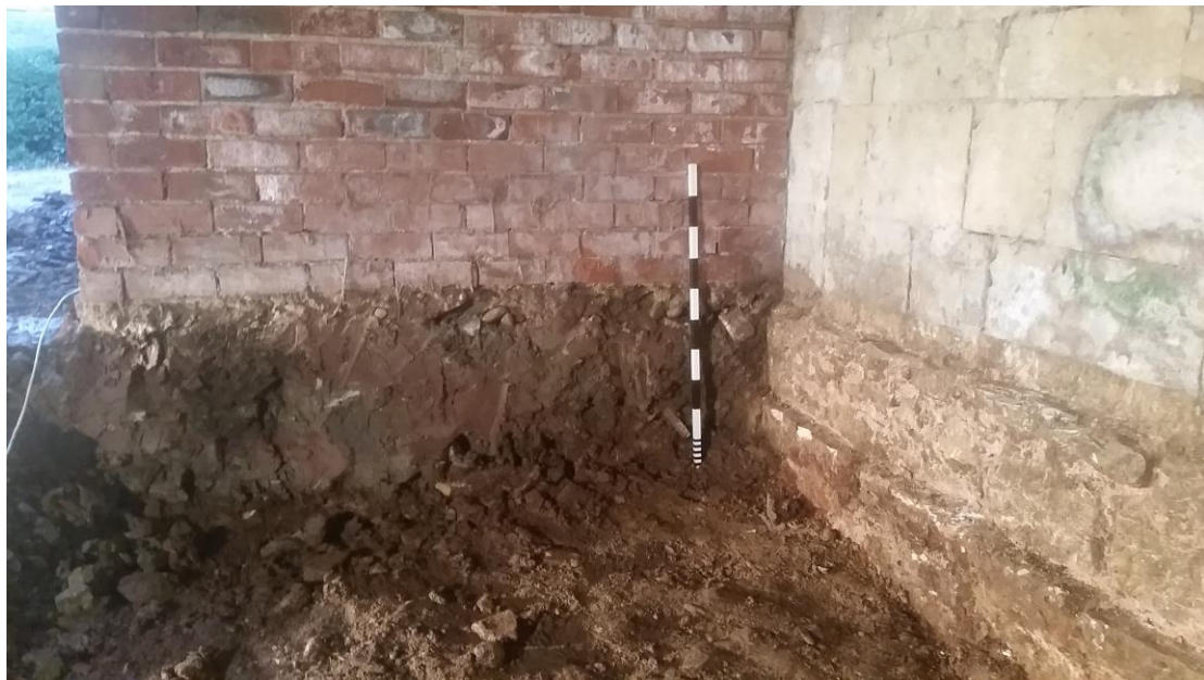
Plate 18 View of construction cut 103 for 105, looking south, 1m scale. Note the stepped nature of 105
