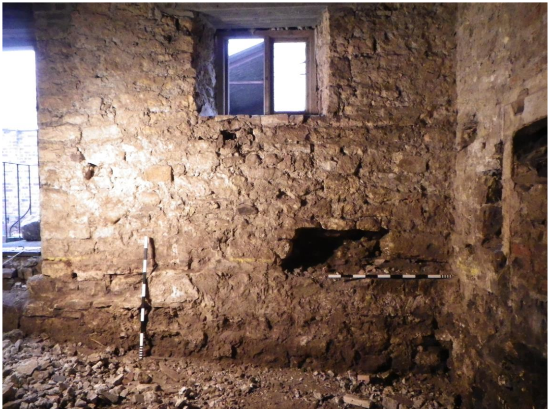
Plate 14 View of the west end of the south wall in the mill interior. Looking south, 1m scales
