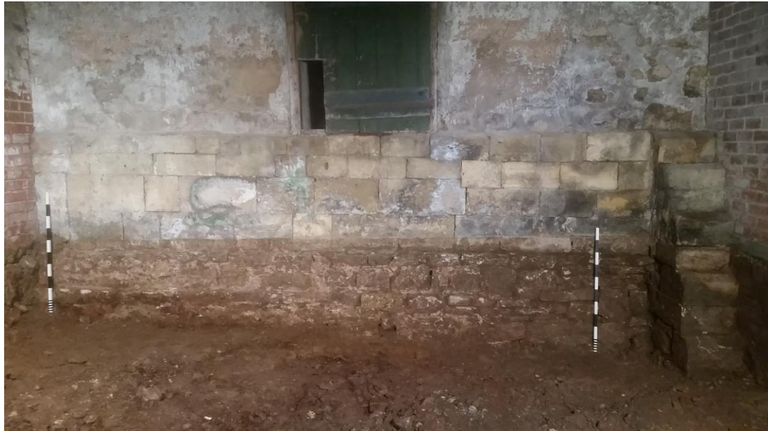
Plate 17 The worked stone foundations 105 for the east exterior wall of the mill, as seen during full depth ground reduction. Reused ashlar blocks 109 may be seen above. Looking west, 1m scales. Note rebuilt supporting buttress 108 to right (north)
