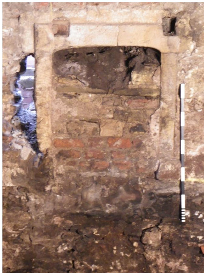
Plate 12 Detail of inserted fireplace 112 in the west wall. Looking west, 1m scale
