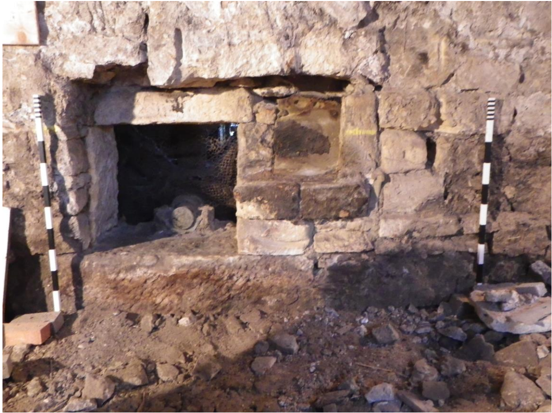
Plate 5 North wall interior, central layshaft and subsequent alterations, looking north, 1m scales
