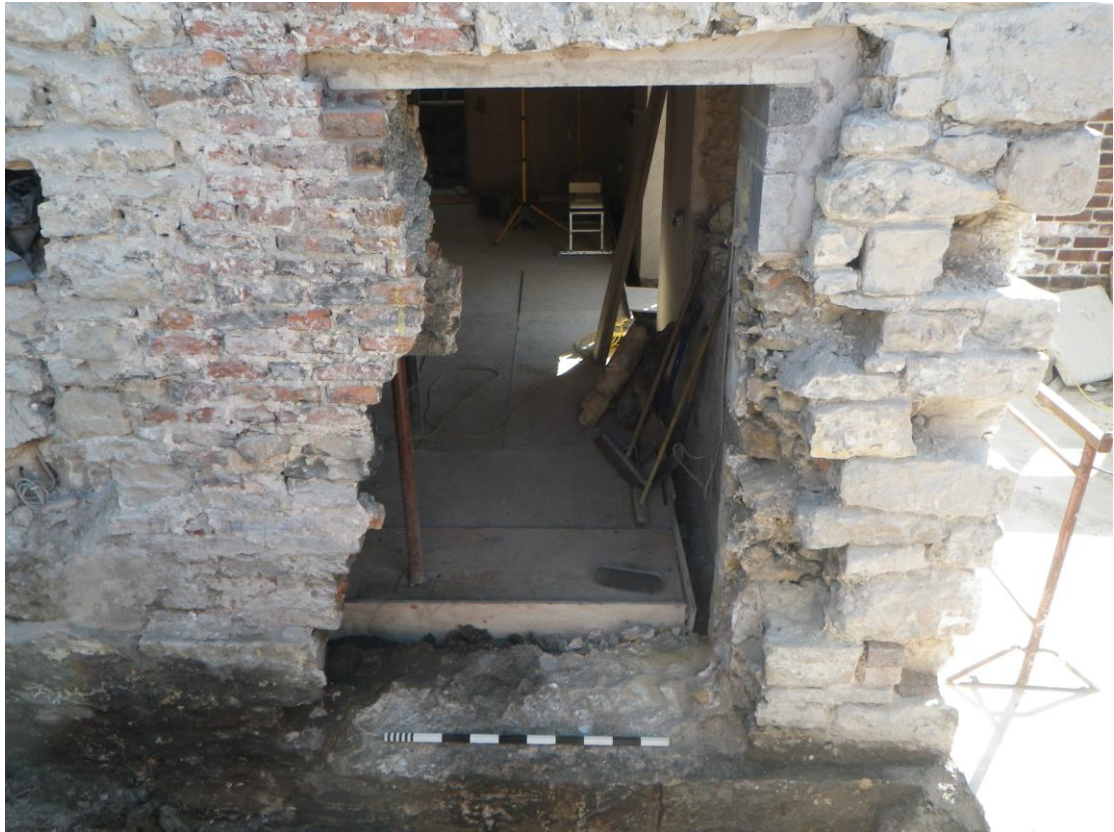
Plate 24 The new entrance into the west side of the mill, looking east, 1m scale
