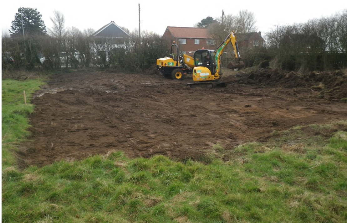
Plate 4 The site undergoing the site strip, only partially removing topsoil 101, looking S
