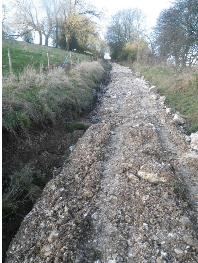
Plate 15 Trench on the south side of the road running down into Thixendale, looking west
