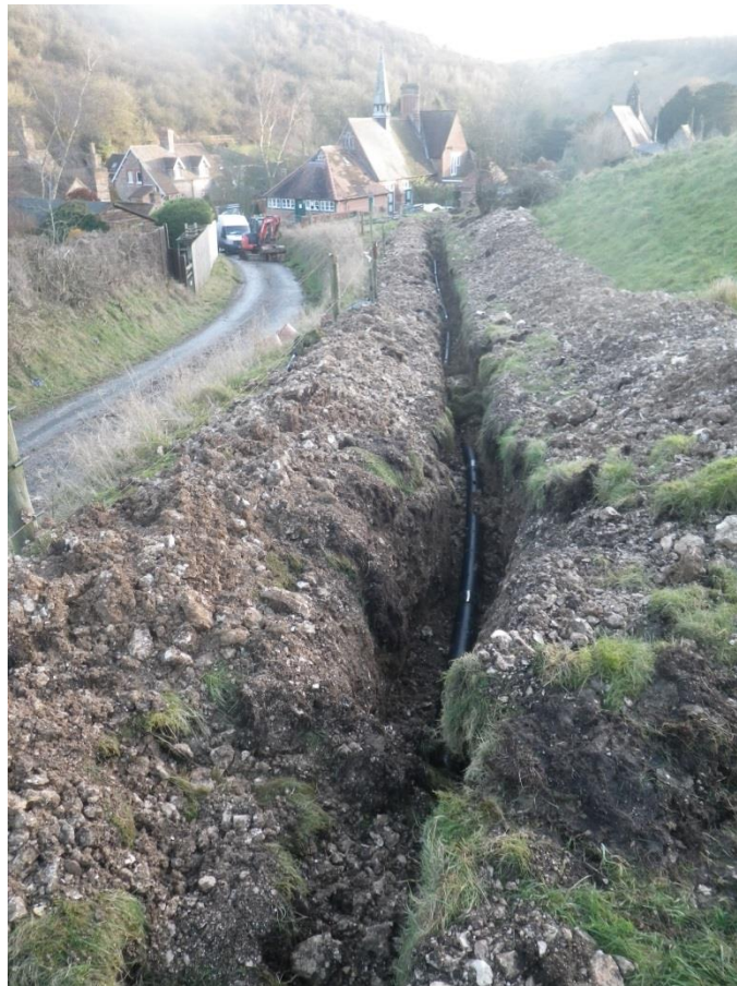
Plate 14 The field C trench running along the north side of the field, looking north-east
