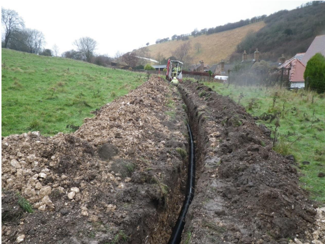
Plate 11 Excavation of the trench continuing to the west in field C, looking north-west
