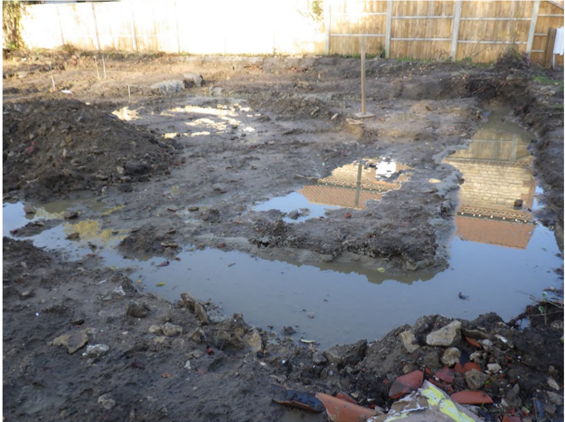
Plate 5 General shot of part of the house foundation at the eastern end, showing poor site conditions.
