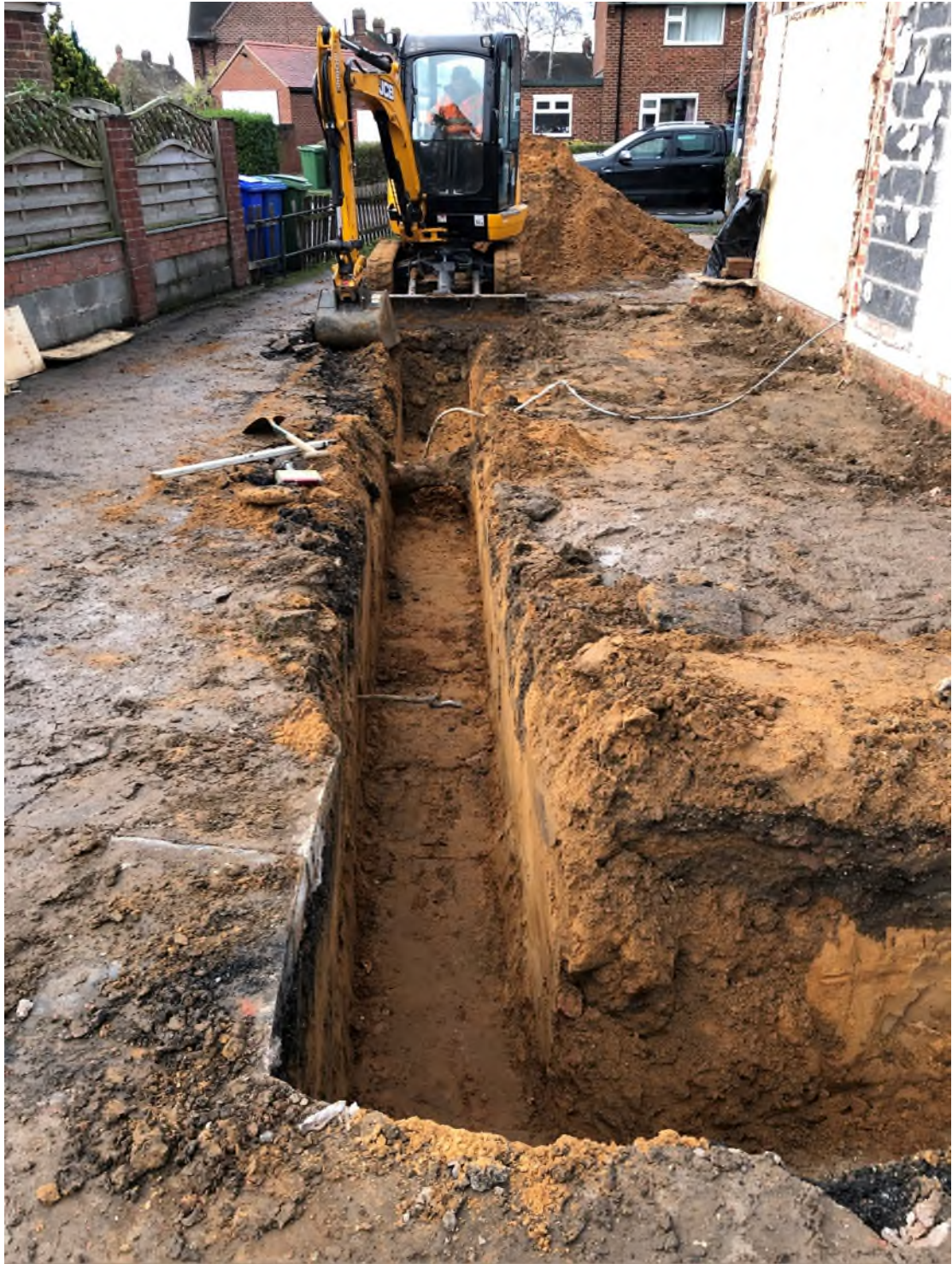
Plate 4 View looking west down the length of the southern foundation trench with the lead water pipes and foul drain crossing the trench
