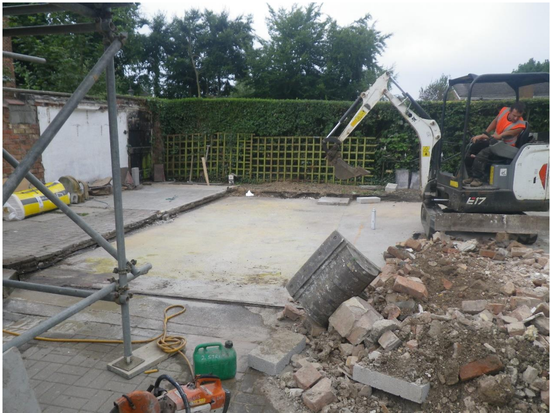
Plate 6 footprint of new garage with recently demolished garage rubble in foreground, looking east
