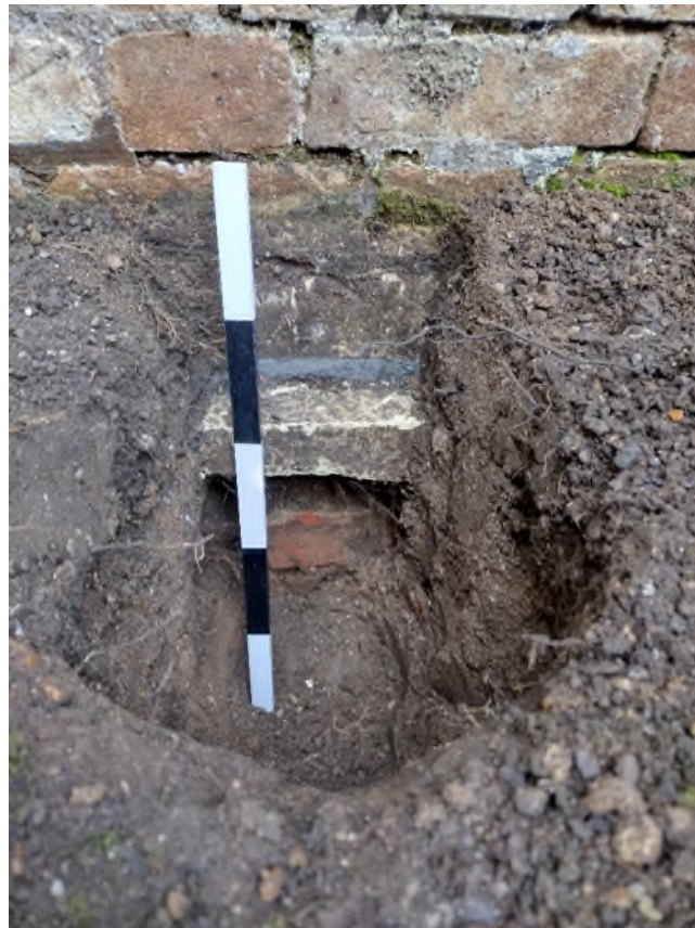
Plate 2 Intervention pit #1 on the eastern side of the north porch, showing likely post-medieval brick footing 103 (red brick, pre-1814) set back and underneath the current north porch foundations 101 (white brick) which was built around 1866. Looking west, 0.5m scale.
