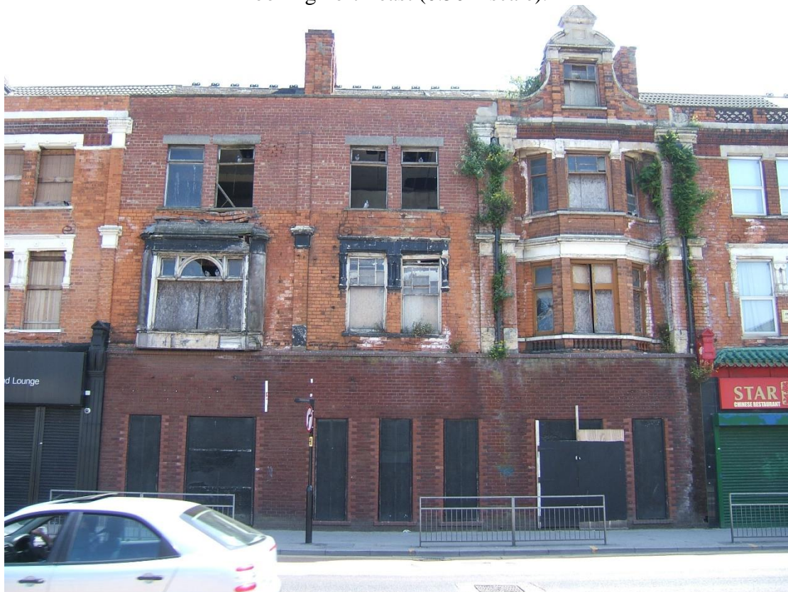
Plate 24 General view of western elevation prior to the addition of scaffolding, looking east.
