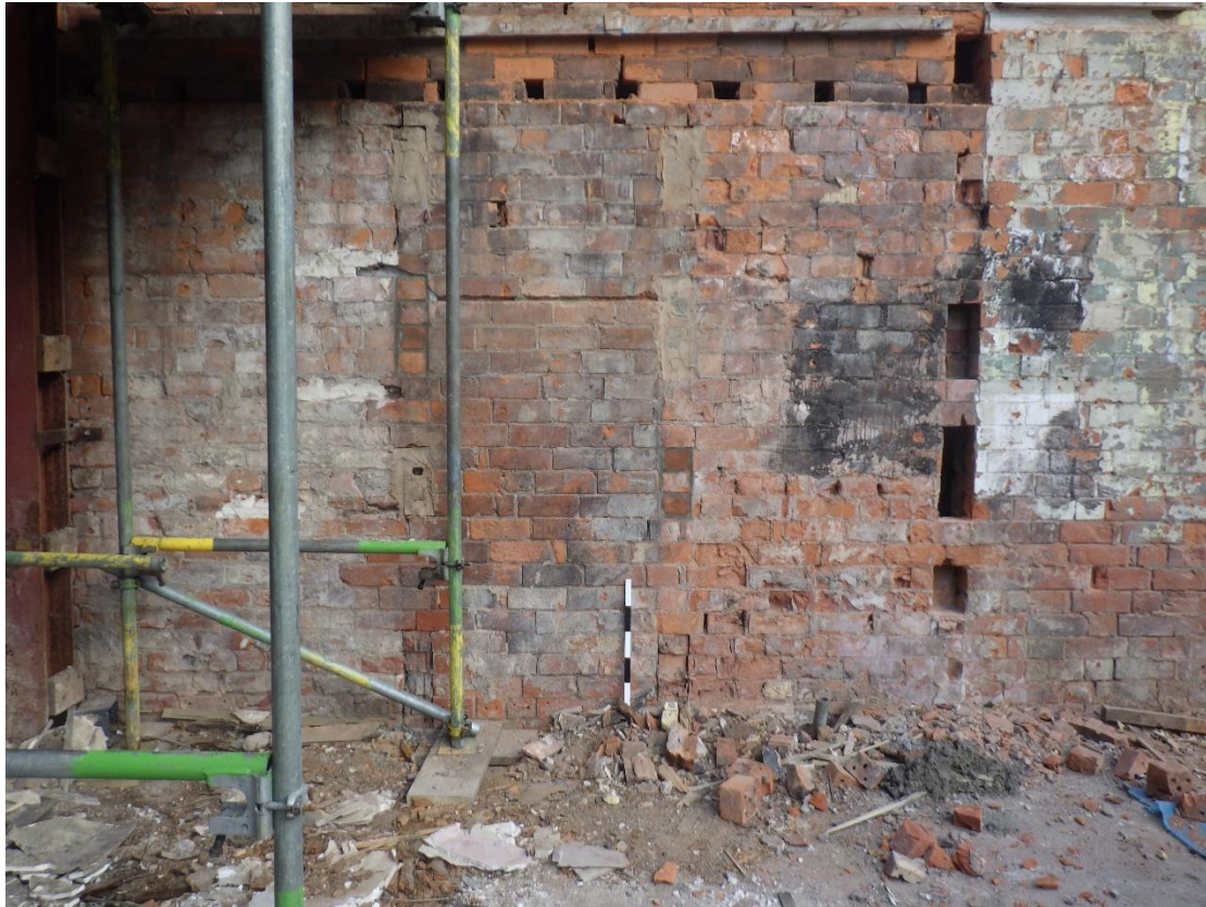
Plate 7 Structural remains showing construction marks from a now demolished portion of the building, looking north (0.50m scale).
