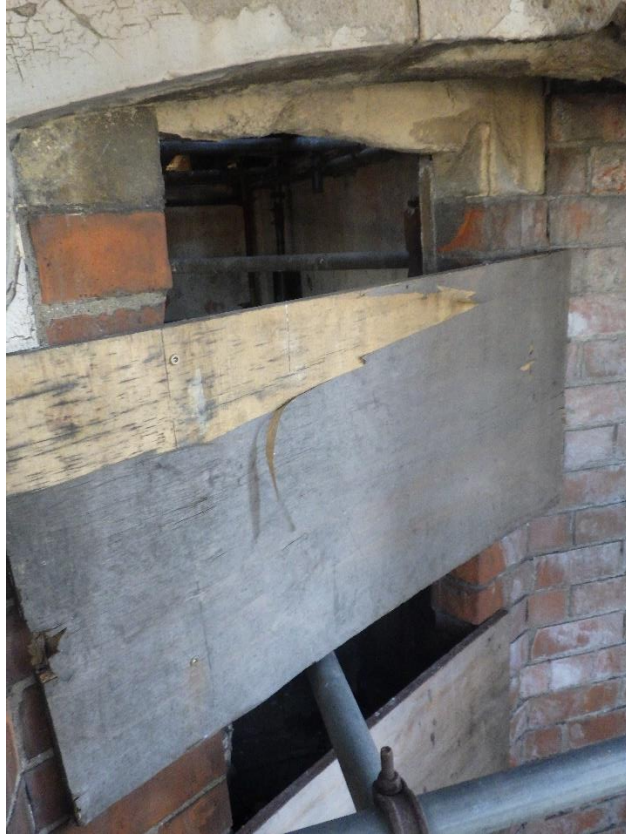
Plate 15 Boarded up window on the southern side of bay window on second storey, looking east.
