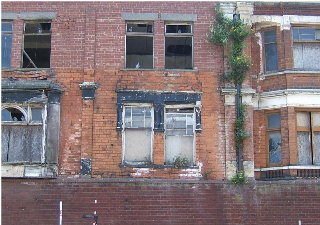
Plate 22 Detail shot of decorative brickwork showing a scrolled pattern between windows on the first storey, looking east.
