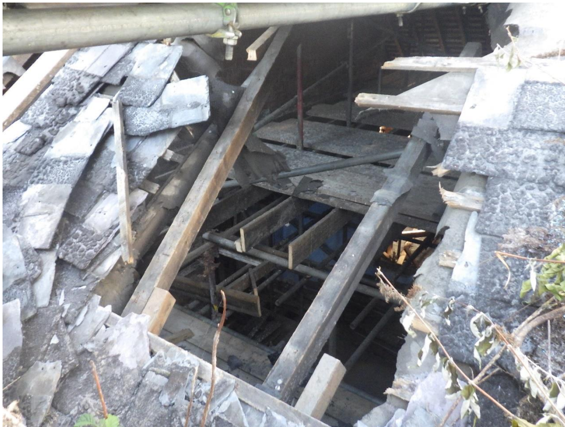
Plate 8 Detail shot of hole in the roof used to facilitate the construction of a scaffold, looking north-east.
