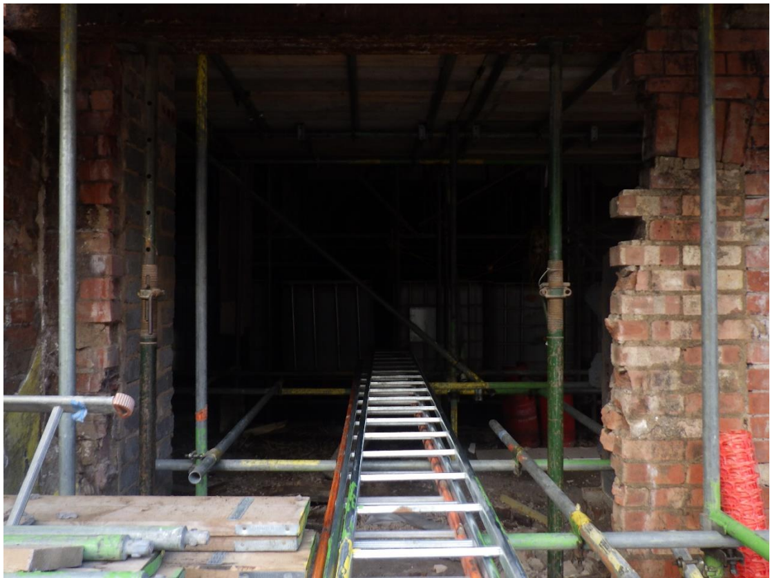
Plate 4 General view of opening on ground floor of eastern elevation, looking west.
