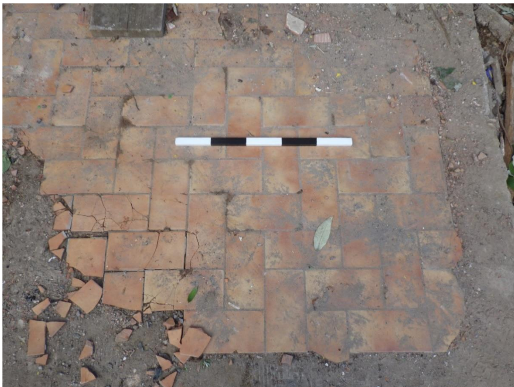
Plate 6 Detail shot of floor tiles on ground floor at rear of the property (0.50m scale).
