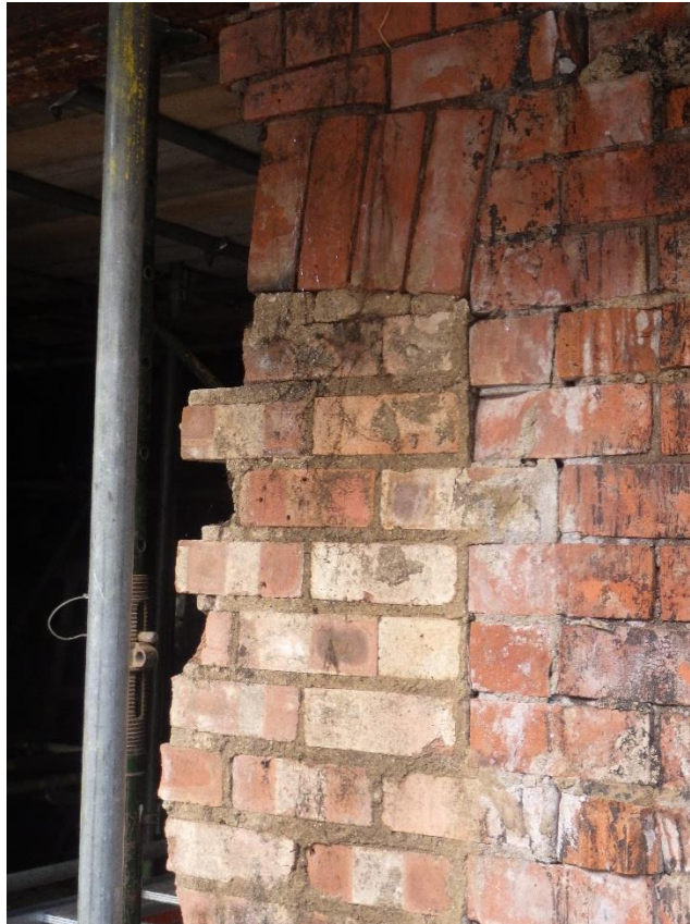
Plate 5 Detail shot of bricked up doorway on ground floor of eastern elevation, looking south-west.
