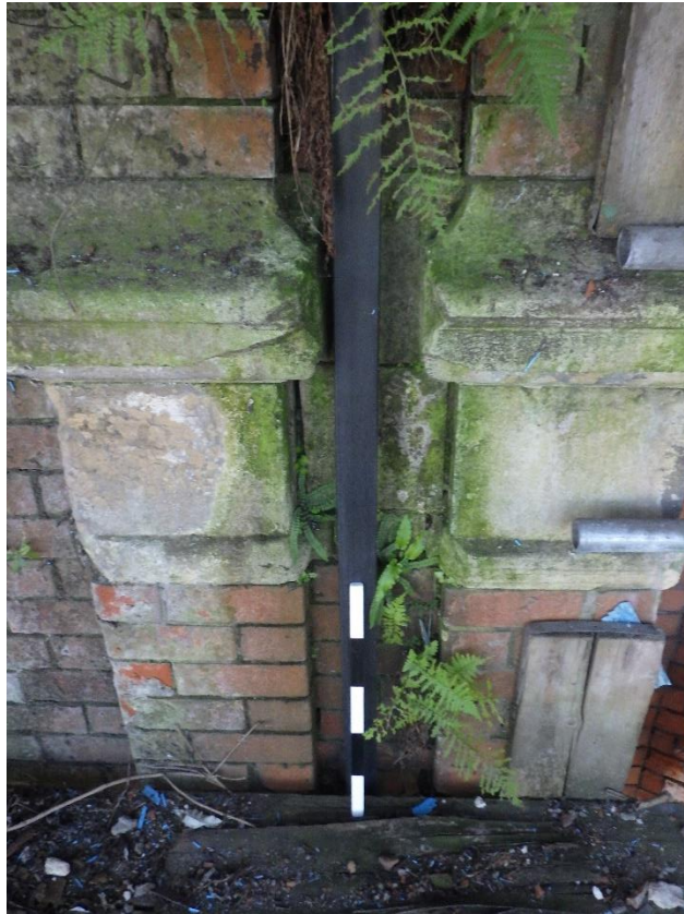
Plate 19 Detail shot of decorative stone capitals on brick columns situated on the western elevation, looking east (0.50m scale).
