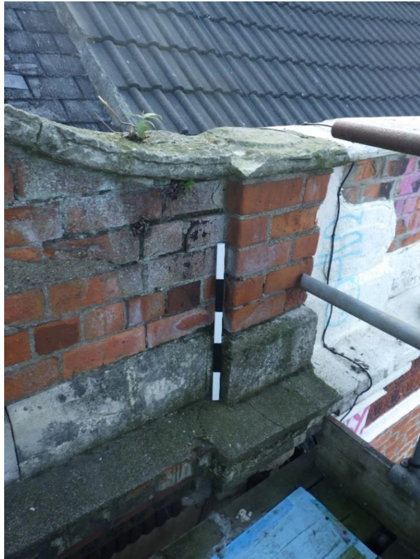
Plate 11 Brick details and end pillar to the south of dormer window, looking south-east (0.50m scale).
