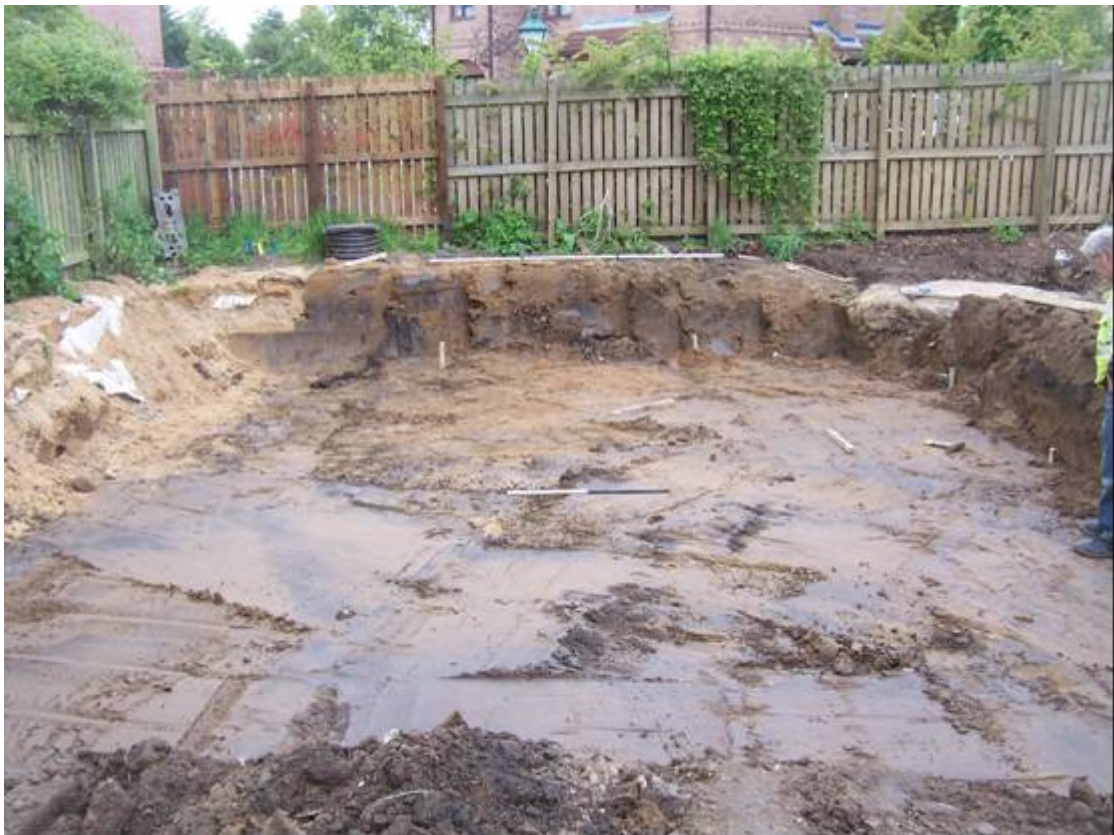
Plate 2 Garage foundations for Plot 3 at the southern end of the site with linear (307) on the left, looking west, 1.00m scale.
