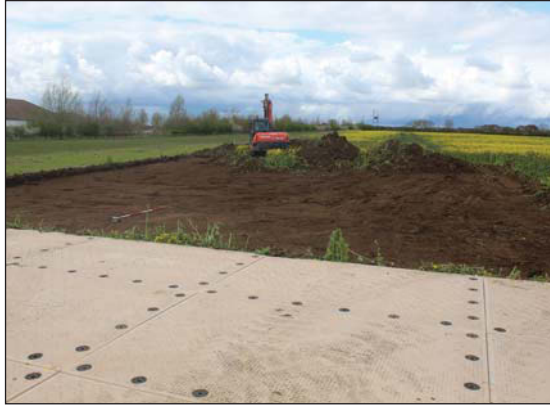
Plate 1. Progress of topsoil strip for compound, looking North, Scales: 2m and 0.5m.
