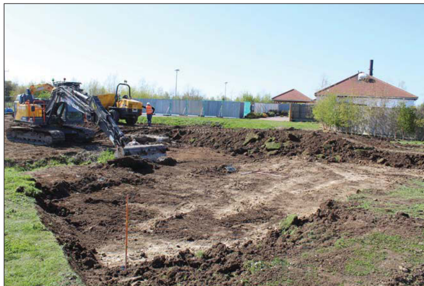
Plate 3. Stripped east end of car park extension, looking North West, Scales: 1m x2.
