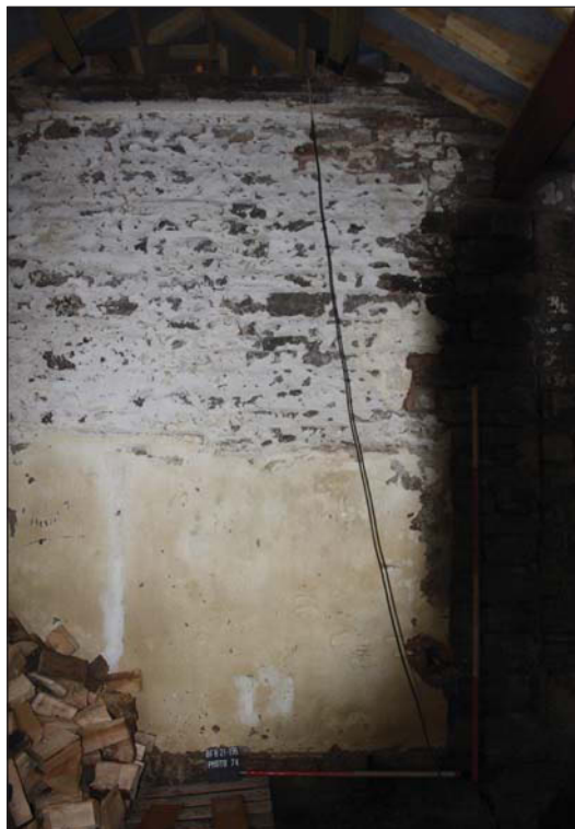
Plate 32. Internal elevation of western wall of stable showing render and limewash looking west, Scales: 2m and 1m
