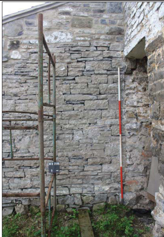
Plate 43. Open coursing on western elevation of lean-to and later opening to cow-house visible right, looking east, Scales: 2m and 1m.
