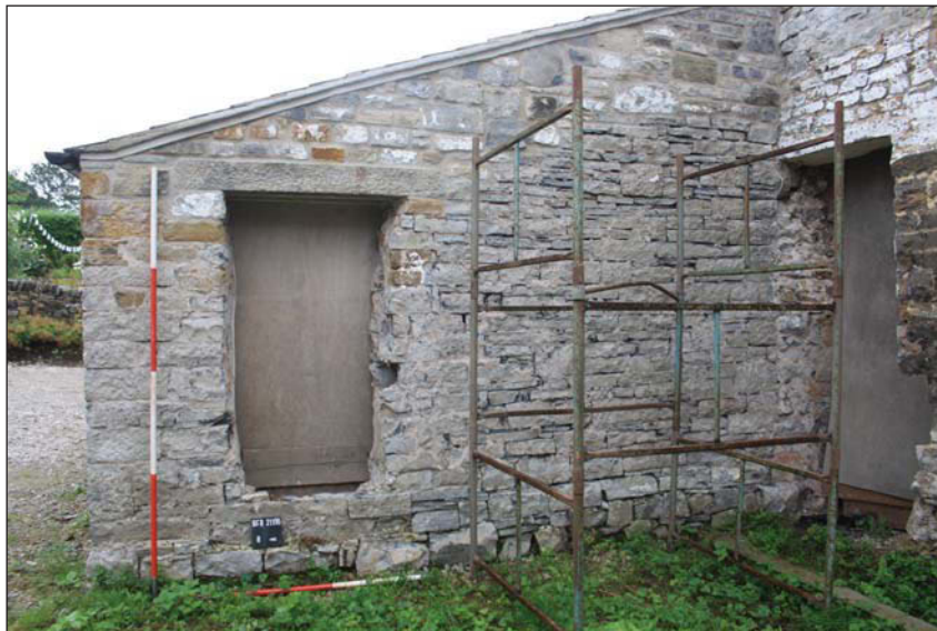
Plate 38. Door or long window in western elevation of lean-to, looking east, Scales: 2m and 1m
