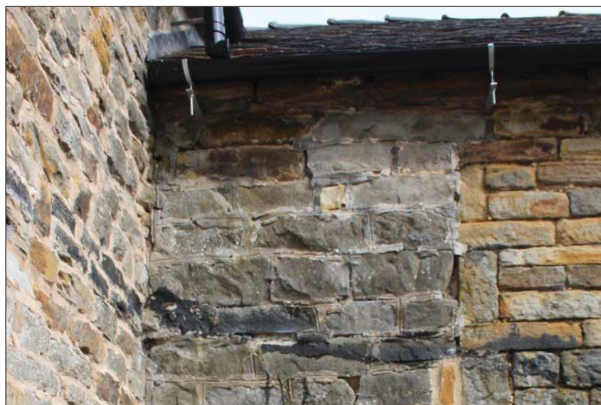
Plate 30. Detail of blocked high-level pitching eye on stable extension abutting the eastern elevation of the cow-house, looking north.
