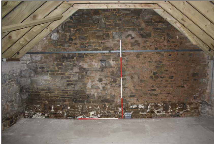
Plate 27. First floor south gable end showing former joist locations, looking south, scales 2m and 1m.
