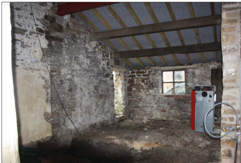
Plate 46. Oblique view of above gable showing interior of lean-to and extent of modern roof replacement on entire structure, looking north-west
