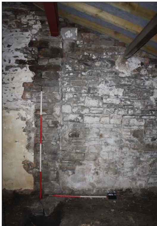
Plate 40. Former location of northern stable wall and steel beam, looking west, Scales: 2m and 1m.
