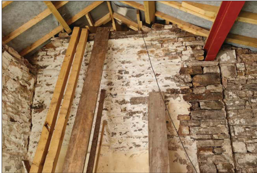
Plate 45. Internal view of previously exterior east gable of cowshed, but now interior and forming west wall of stable, showing straight joints where stable and later lean to attach, looking west.
