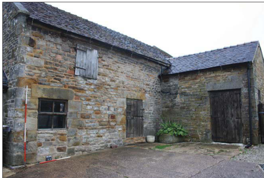
Plate 1. View of eastern elevation of cowhouse and southern elevation of stable, looking north-west,
