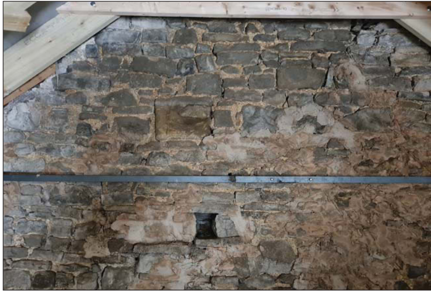
Plate 13. Internal view of repair detail in southern gable of cow-house, looking south.
