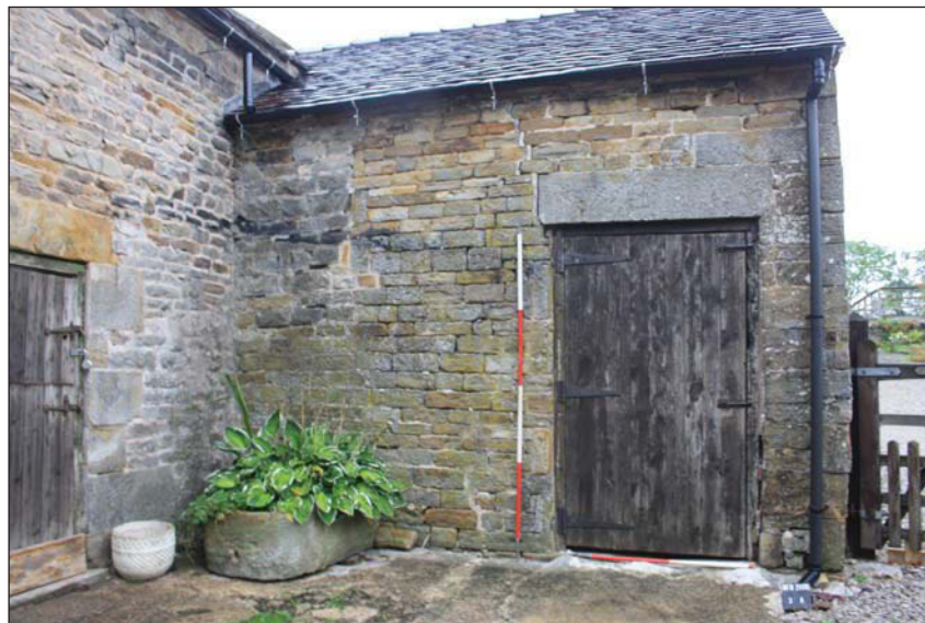
Plate 29. Southern stable elevation with blocked high-level pitching eye abutting the cow-house, looking north, Scales: 2m and 1m
