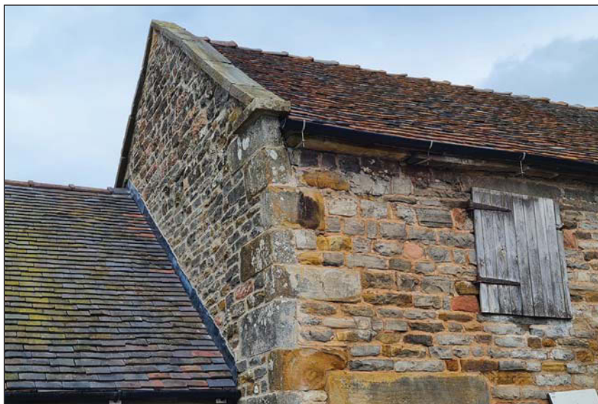
Plate 12. External view of south gable showing location of repair detail, looking west.
