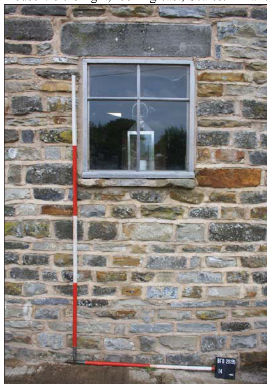
Plate 44. The replacement window and original lintel in the western elevation of cowhouse, looking east, Scales: 2m and 1m.
