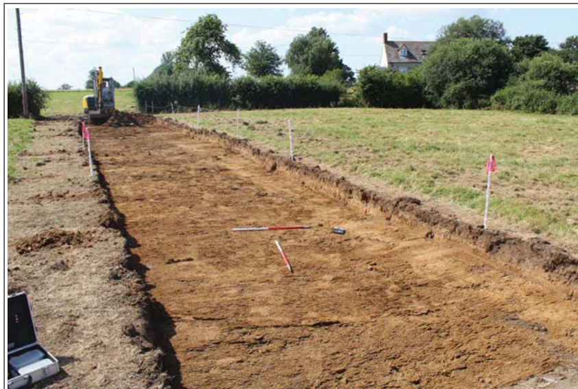
Plate 2. Western portion of new access towards Middle Green Farm, looking North West, Scales: 1m x2, vertical 0.3m.
