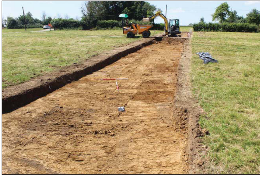
Plate 3. Eastern portion of new access from Baulking Lane, looking West, Scales: horizontal: 1m x2, vertical 0.3m.
