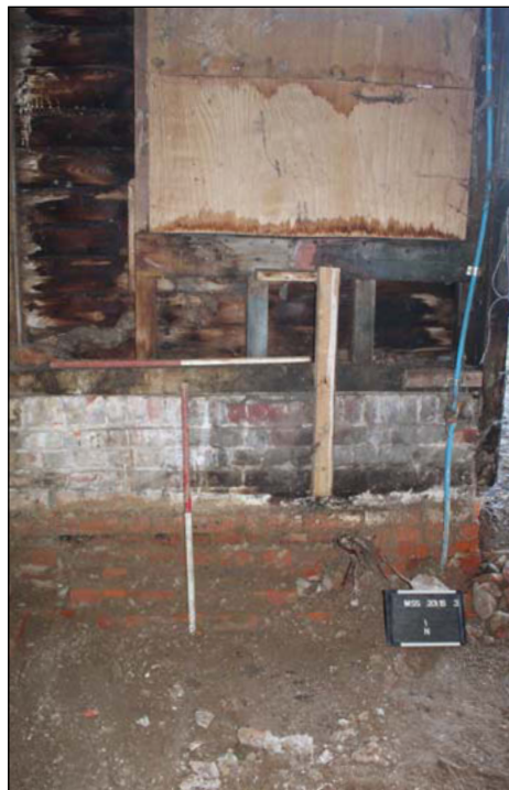
Plate 8. Room C, exposed footing under timber facing, looking South, Scales: horizontal 1m, vertical 1m.
