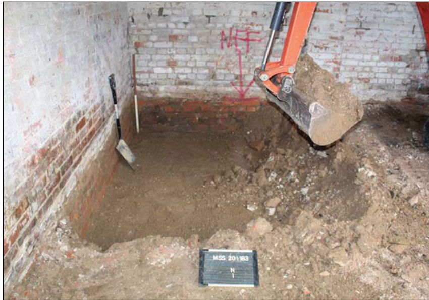
Plate 7. Room C, reduction of north west side of floor in progress, looking North, Scale: 1m.
