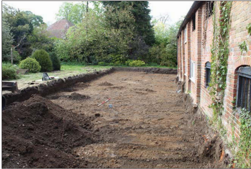
Plate 1. View over stripped area for rear terrace, looking South West, Scale: 2m.
