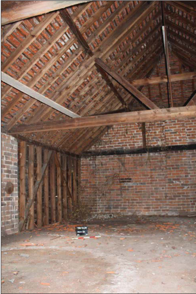
Plate 13. Room 5, General view and oblique of truss and roof detail, looking North West; Scale 0.5m.
