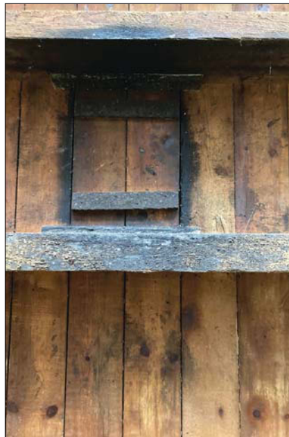
Plate 35. Garage, evidence of burning in the ceiling, looking up.
