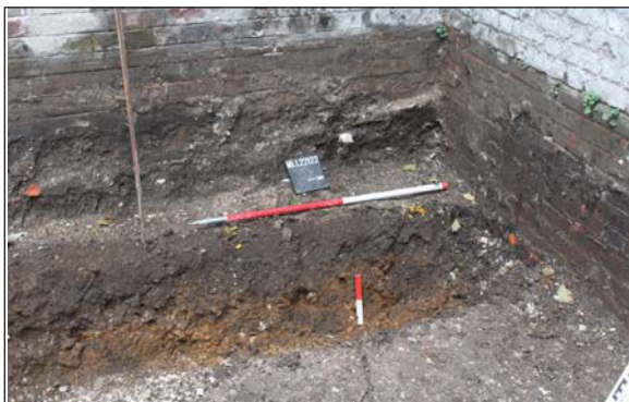
Plate 5. Footing trench in North-west corner of site (following initial ground reduction), looking North-West. Scales: 1m and 0.20m.
